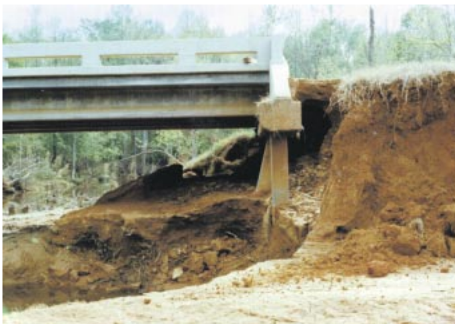
Figure 1. An example of bridge-abutment scour in central Mississippi.
