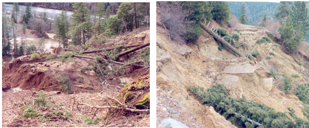
Figure 2 Slump South Fk Salmon River (left); Earthflow on road, Walker Creek (right).
