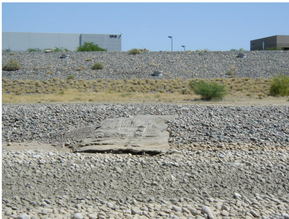
Figure 6 Exposed guide dike following the February 2005 event.
