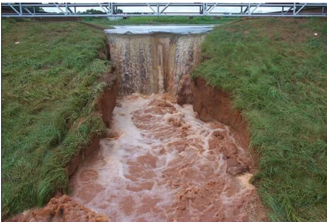
Figure 1 Observed gully erosion during embankment overtopping test.
