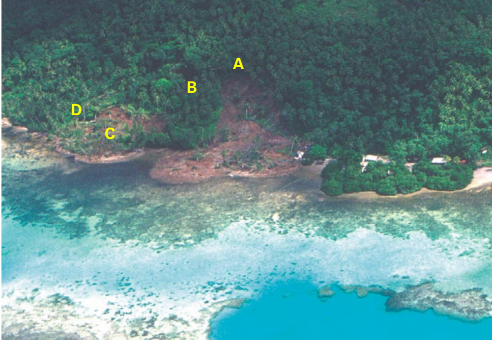
Figure 21. Aerial view of the Faia landslide and incipient slumps. Letters denote locations described in text.
