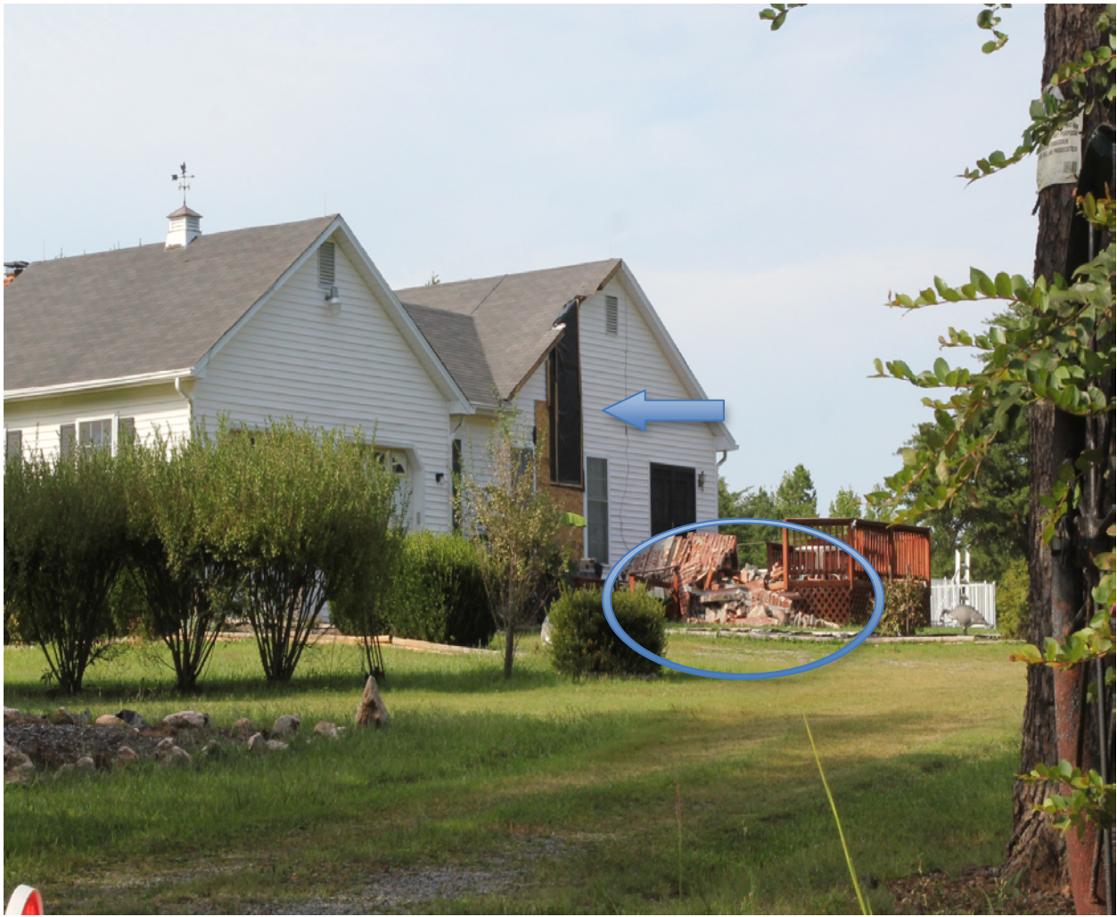
Figure 14. Photograph of a Louisa, Virginia, residence with a collapsed chimney after the August 23, 2011, Mineral, Virginia, earthquake. Arrow indicates the exposed black tarpaper on the side of this house where the chimney stood before the earthquake. The oval indicates the pile of rubble left after the chimney fell down.
