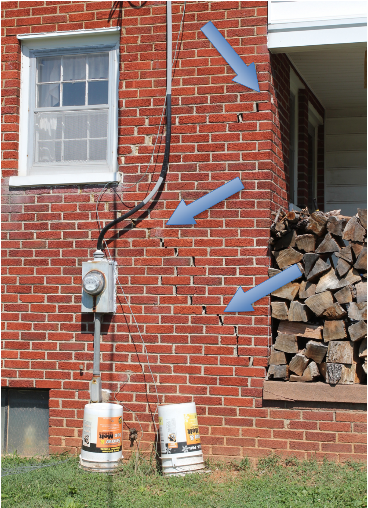
Figure 12. Photograph of a cracked brick wall at a Mineral, Virginia, residence after the August 23, 2011, Mineral, Virginia, earthquake.
