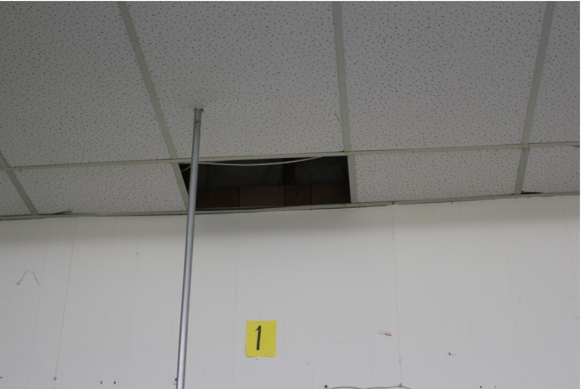
Figure 7. Photograph of a fallen ceiling panel in the local Mineral, Virginia, grocery store after August 23, 2011, Mineral, Virginia, earthquake.
