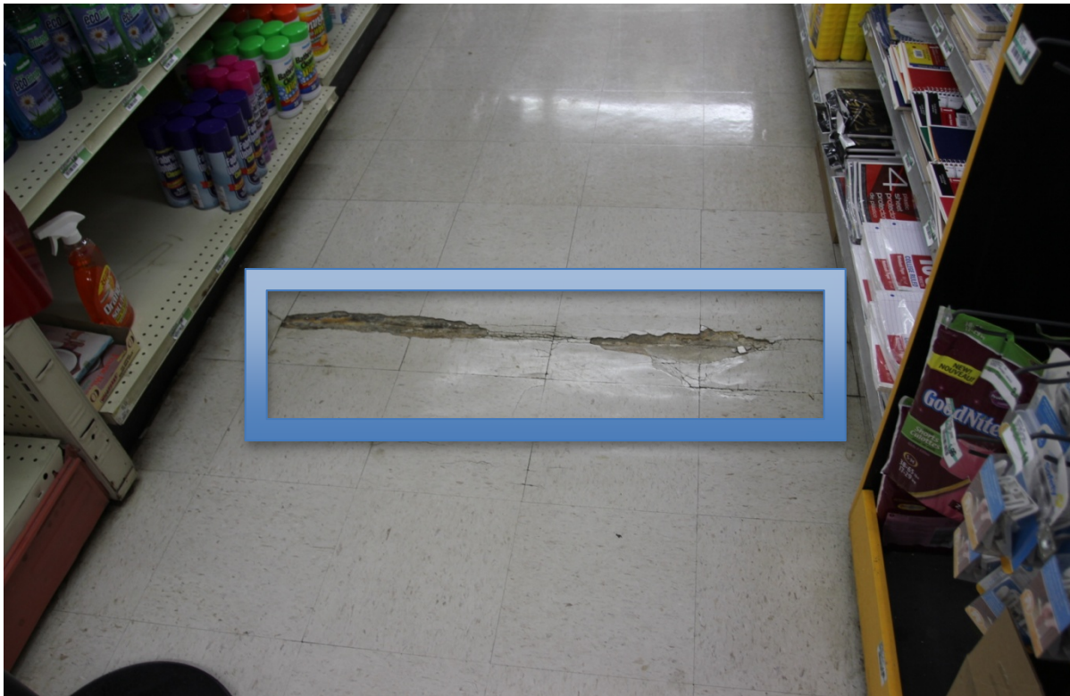
Figure 8. Photograph of one of several large floor cracks (outlined by blue rectangle) in the local Mineral, Virginia, grocery store after August 23, 2011, Mineral, Virginia, earthquake.
