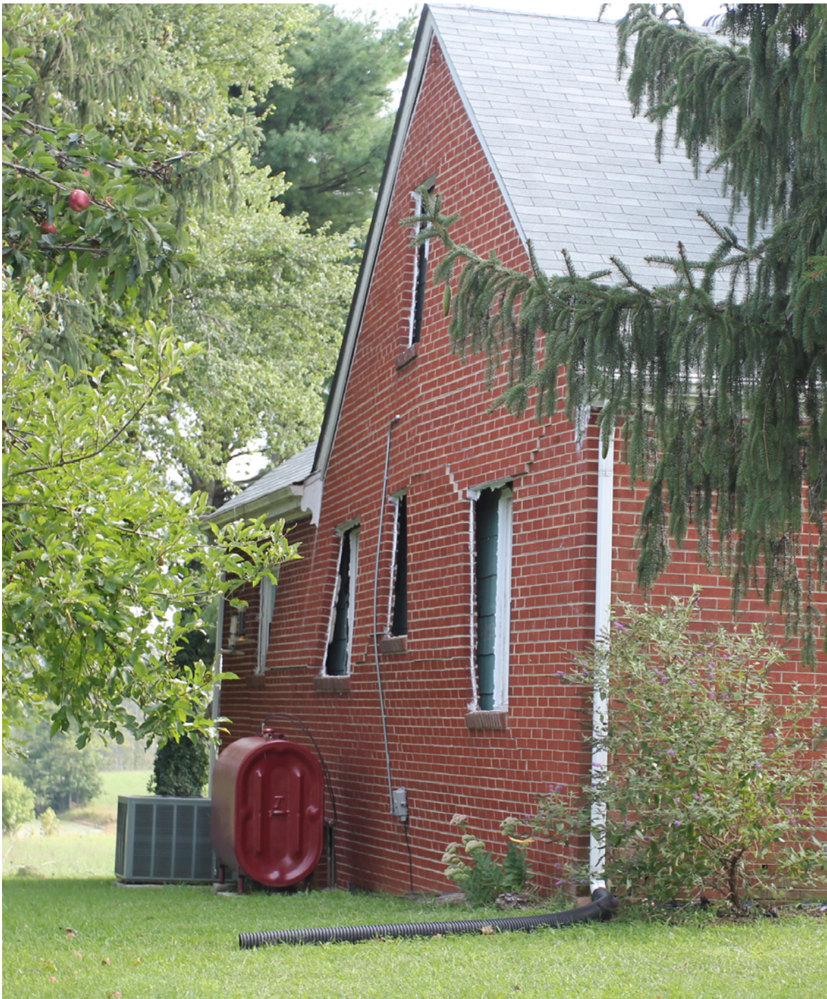
Figure 17. Photograph of a brick wall of a Louisa, Virginia, residence after the August 23, 2011, Mineral, Virginia, earthquake. The wall was damaged in the earthquake and can clearly be seen bowing away from the main structure. The wall collapsed completely a few days after this photo was taken.
