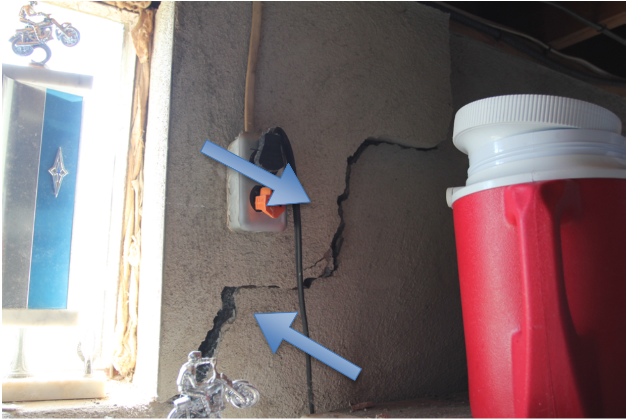
Figure 9. Photograph of a crack in the basement of a Mineral, Virginia, residence after the August 23, 2011, Mineral, Virginia, earthquake. Image shows “stair-stepping” (bottom left to upper right) under the electrical outlet, approximately 0.5 meters visible here.
