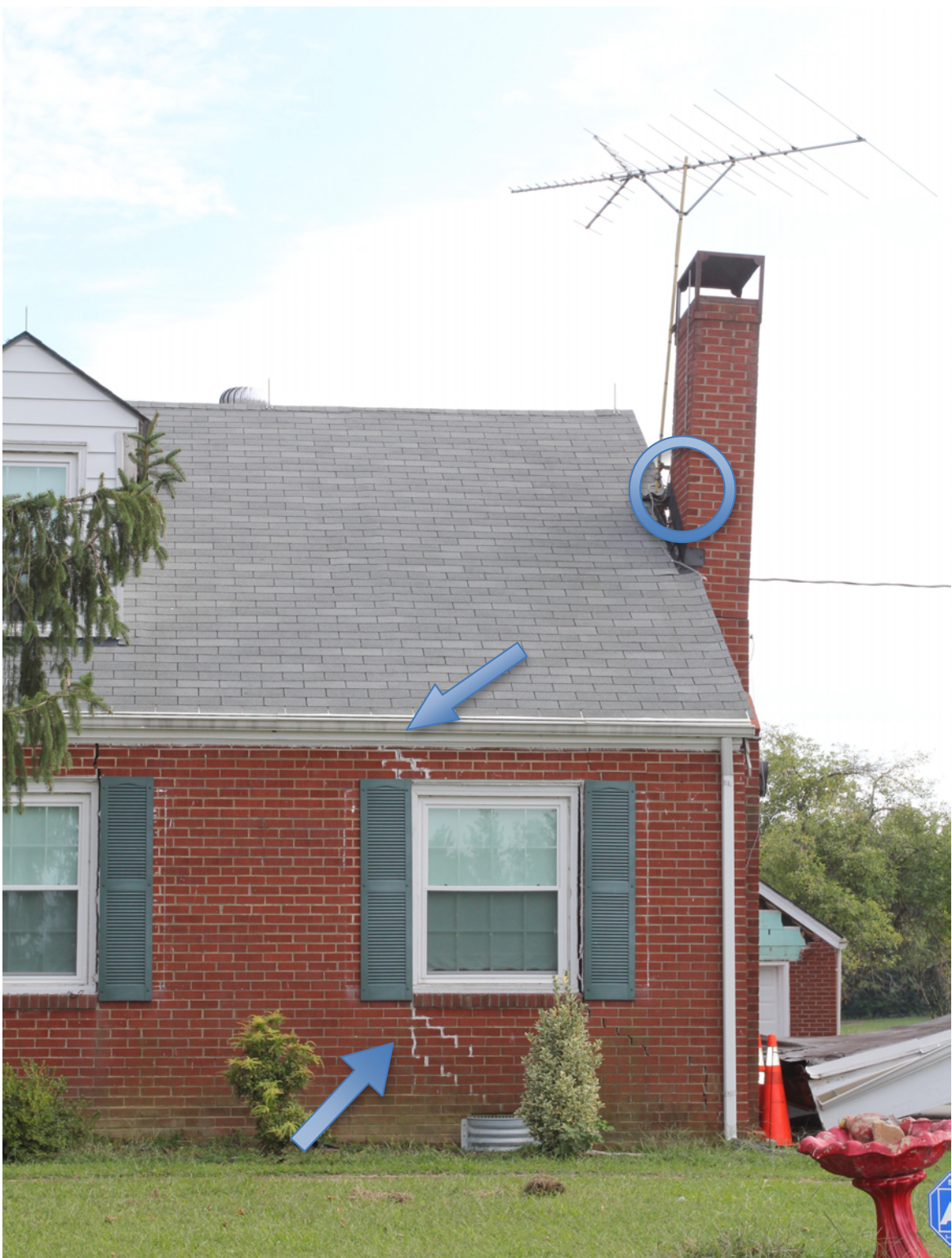
Figure 15. Photograph of a Louisa, Virginia, residence with cracked walls after the August 23, 2011, Mineral, Virginia, earthquake. Blue arrows point at the white cracks stair-stepping along the wall and circle indicates the gap from the leaning chimney; separations from the roof can be seen as the white light between roof and chimney.
