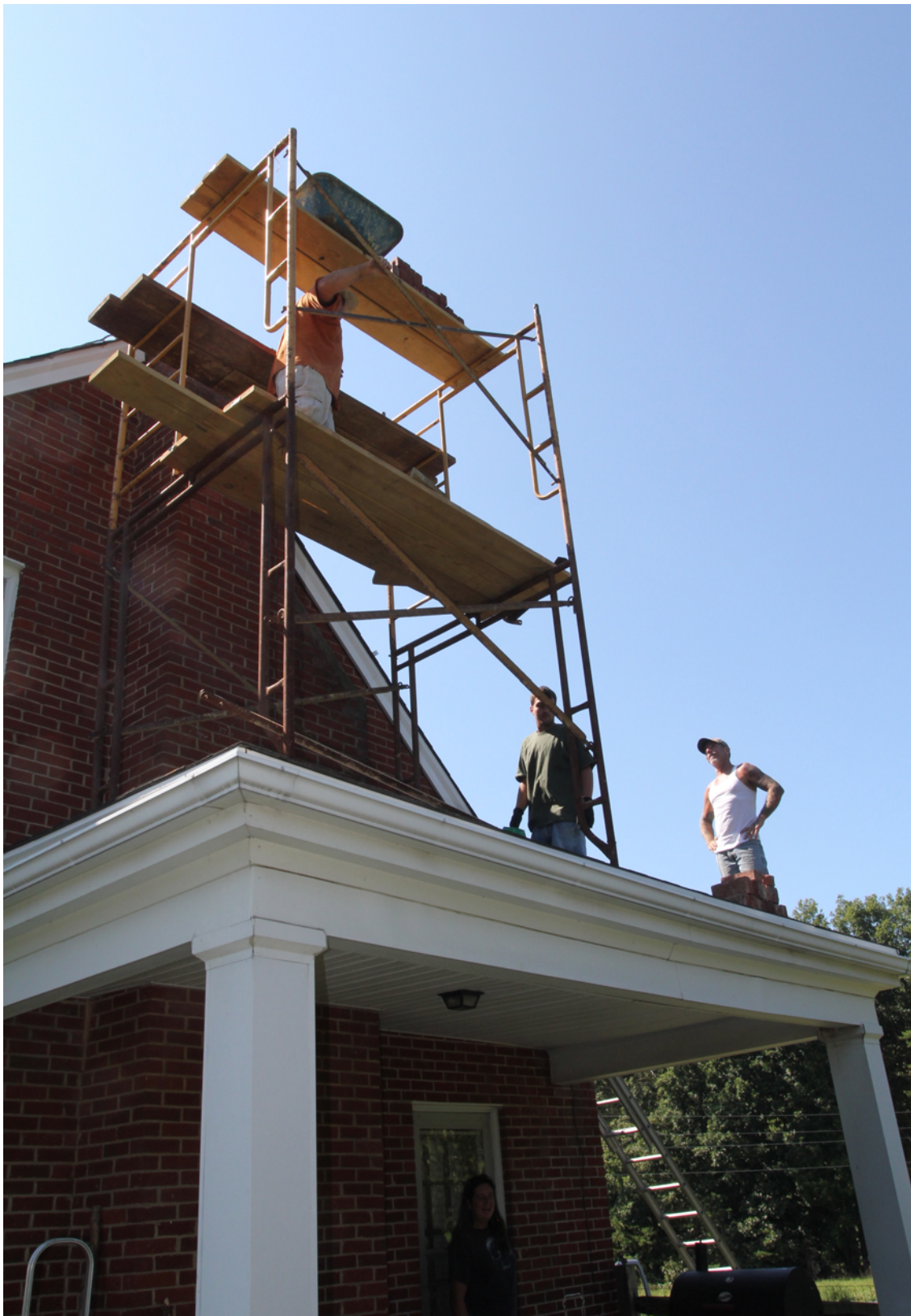
Figure 11. Photograph of chimney repairs beginning on a Mineral, Virginia, residence 7 days after the initial shock of the August 23, 2011, Mineral, Virginia, earthquake.
