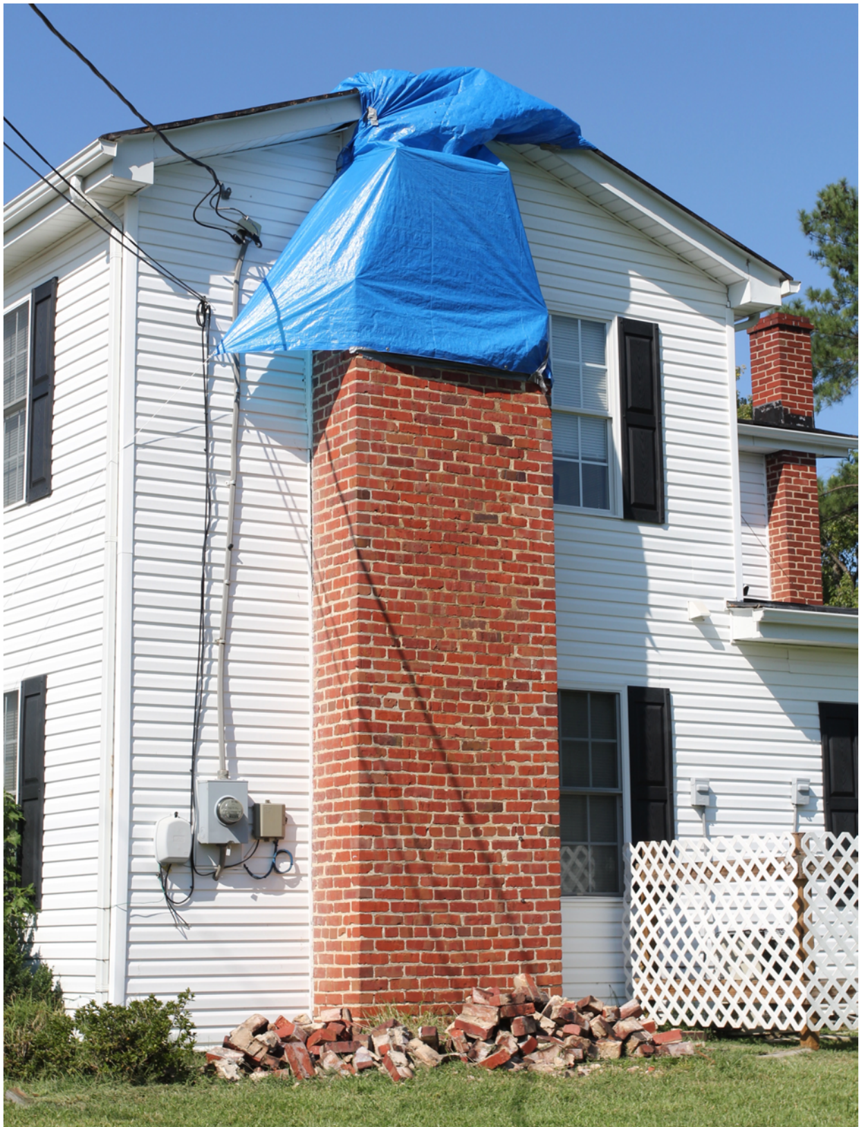
Figure 10. Photograph of broken upper chimney under blue tarp at a Mineral, Virginia, residence after the August 23, 2011, Mineral, Virginia, earthquake. Note the chimney in the right side of the background does not have any visible damage.
