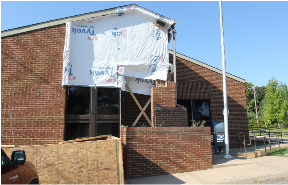
Figure 6. Photograph of the brick façade of the U.S. Post Office in Mineral, Virginia, which collapsed during the August 23, 2011, Mineral, Virginia, earthquake.
