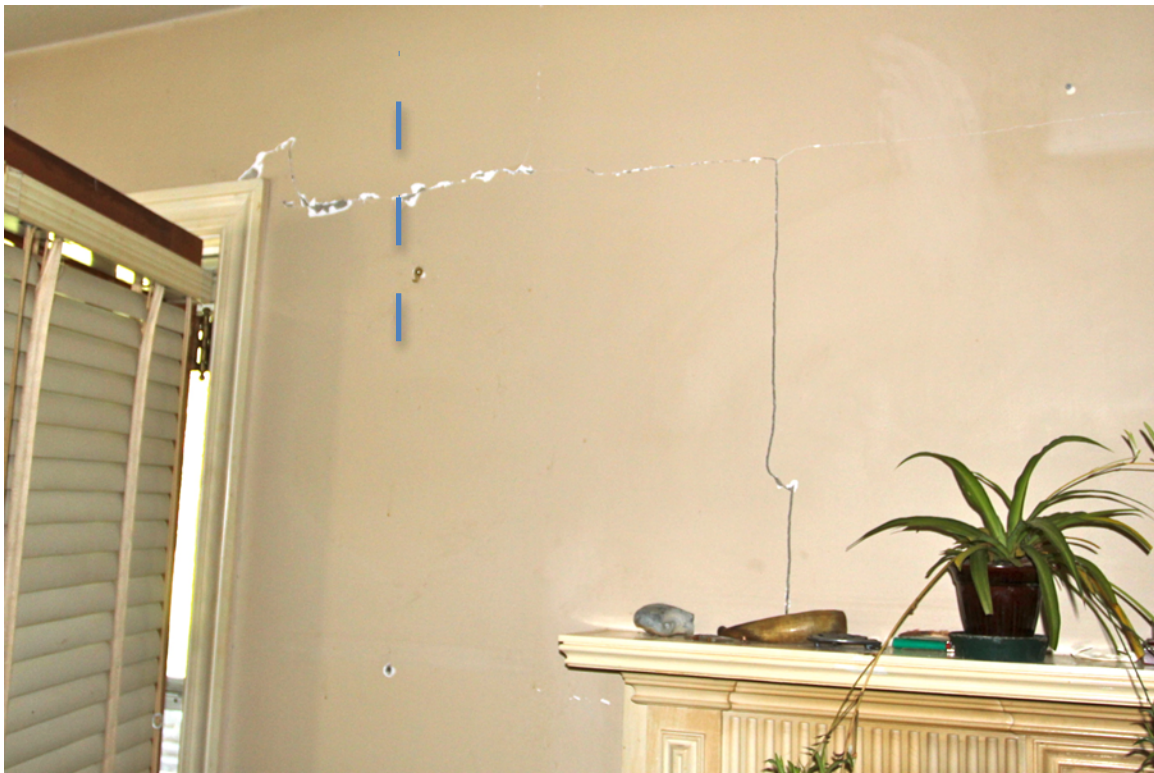
Figure 13. Photograph of cracks in the interior drywall of a Mineral, Virginia, residence after the August 23, 2011, Mineral, Virginia, earthquake. The initial shock caused the crack to extend from the corner of the doorframe to the blue dashed line. All of the cracks emanated to the right and down. Cracks to the right of the blue dashed line occurred during aftershocks. Photograph taken 8 days after initial shock.
