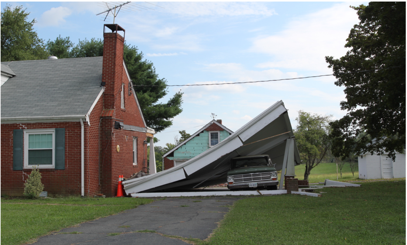
Figure 16. Photograph of the Louisa, Virginia, residence shown in figure 15. The carport shown in the image detached from the house and collapsed as a result of the August 23, 2011, Mineral, Virginia, earthquake, crushing the vehicle underneath it.
