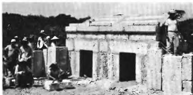
FIGURE 47.—Construction with Ryukyu Limestone. Sandy Ryukyu Limestone is quarried, allowed to harden, and used in the construction of native tombs, walls of buildings, and retaining walls. The tomb in the picture is being constructed of blocks of sandy Ryukyu Limestone locally called awaishi. October 1956.
