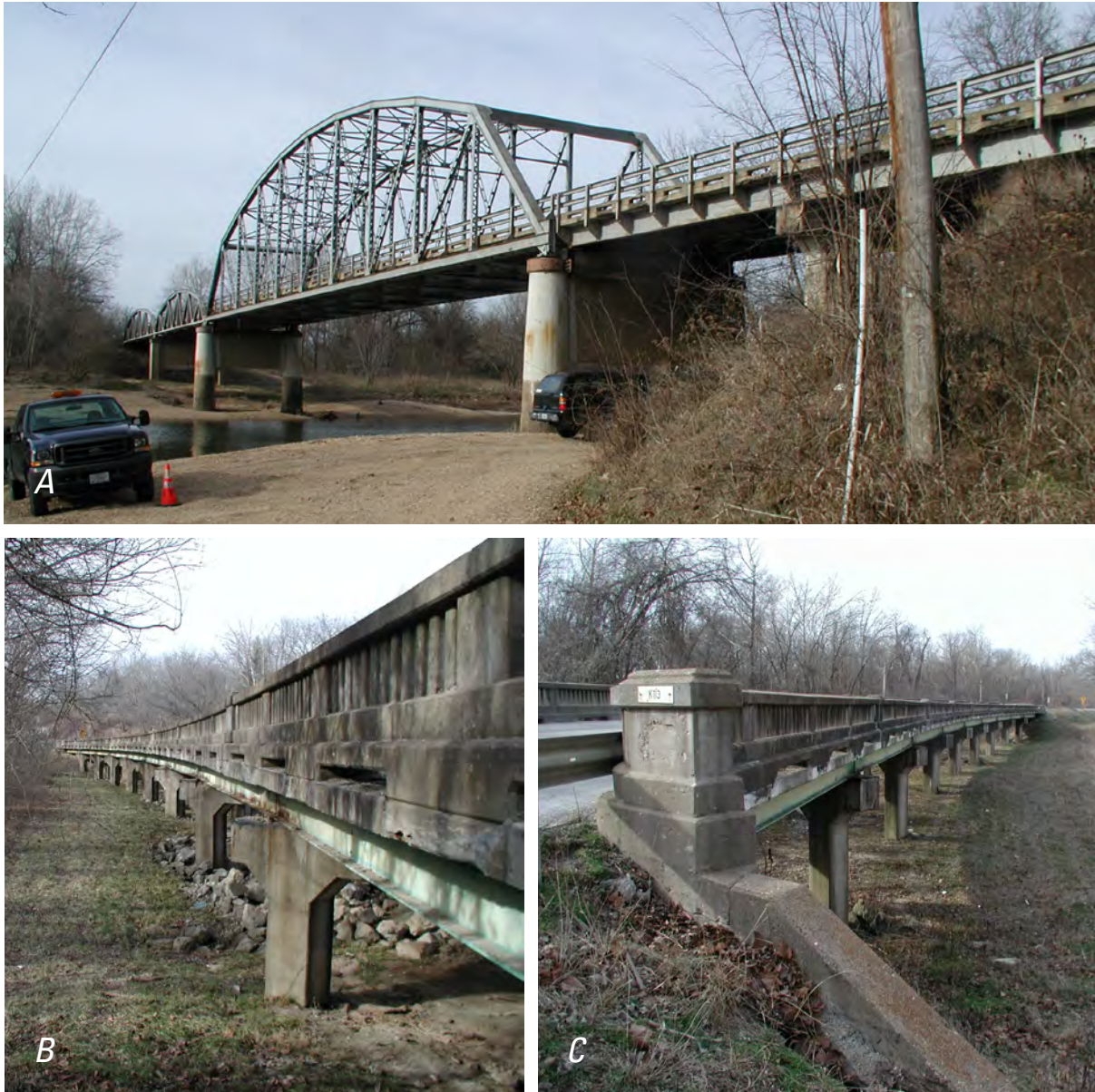
Figure 5. State Highway 17 crossing of the Gasconade River near Waynesville, Missouri, on January 4, 2008; A , Upstream face of main channel structure J-802, spanning the gravel bed of the river, as viewed from the right bank immediately upstream from the right (east) abutment at the base of a limestone and dolomite bluff, B , upstream face of left (west) overflow structure K-112, as viewed from the upstream top of the right (east) abutment; and C , downstream face of middle overflow structure K-113, as viewed from the downstream top of the right (east) abutment.
