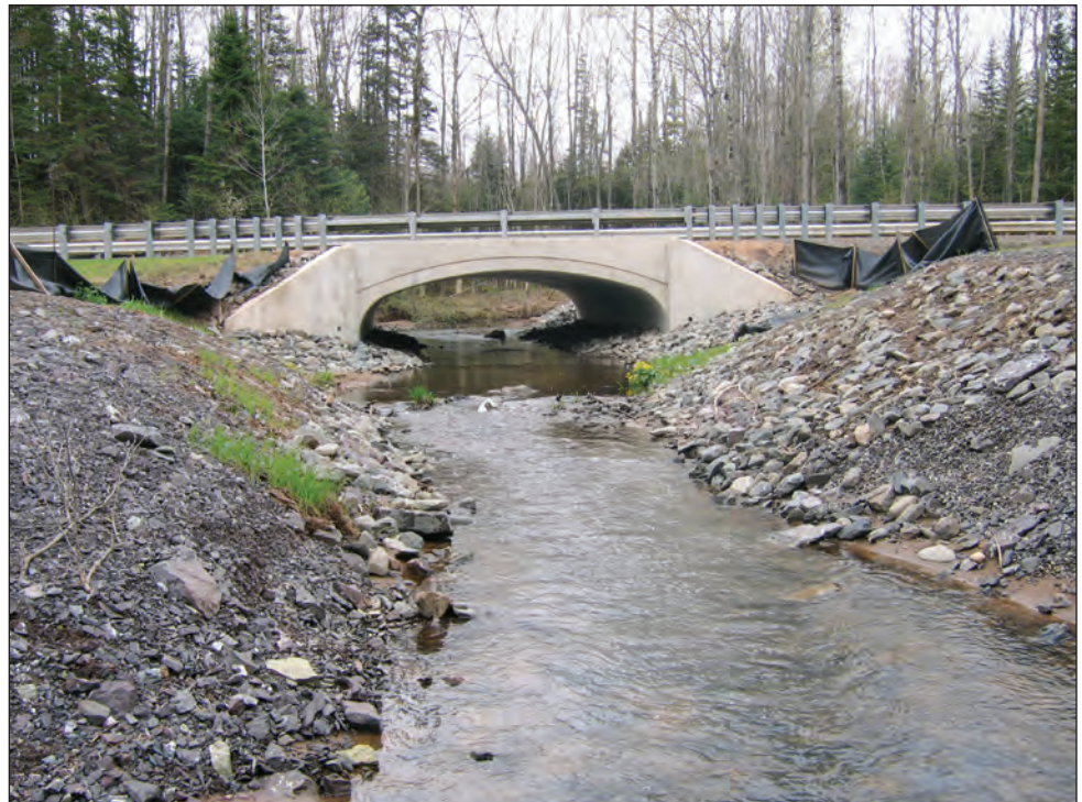
Figure 12. View looking upstream at a concrete culvert at the Indian Road crossing of Gomanche Creek (U.S. Geological Survey streamgage 04043140), May 11, 2005. (Photograph by T.L. Weaver U.S. Geological Survey)
