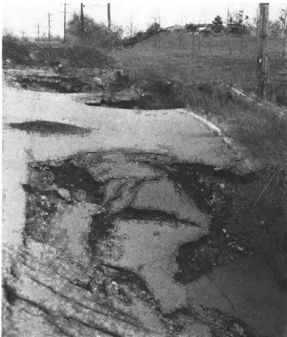
Figure 6.--Collapse beneath State Route 29, 1 mile north of U.S. Route 202.
