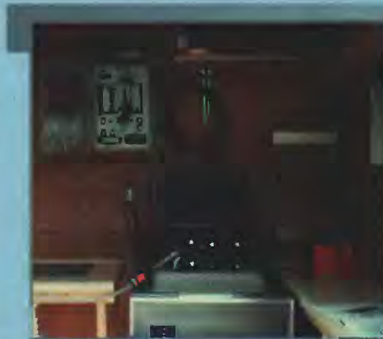
Figure 4. Automatic sampling equipment at each site includes a flow meter for continuously recording discharge and a refrigerated automatic sampler for collecting and preserving water samples.
