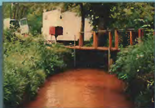
Figure 3. Housing was installed at each monitoring site to protect automatic sampling equipment and to allow automated water-quality sampling during high-flow events.
