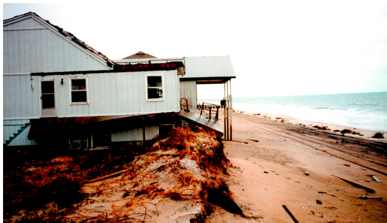
House at Topsail Beach now located seaward of dunes after Hurricane Floyd
