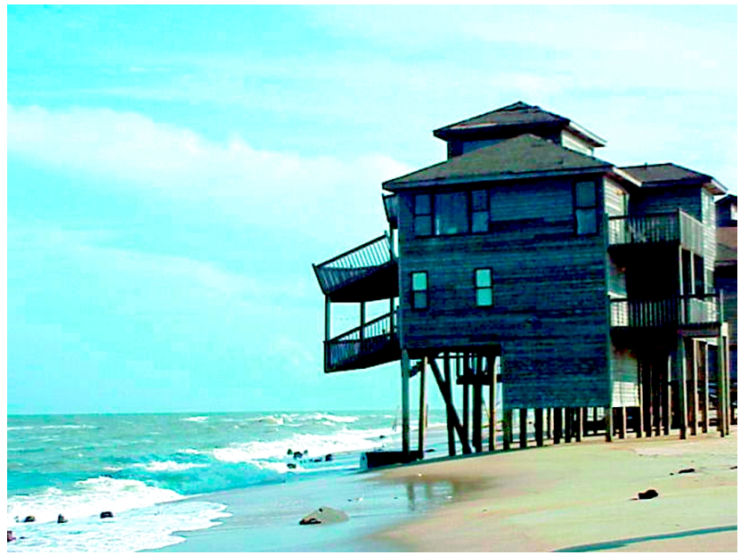
Figure 27. Houses standing in the surf at Rodanthe, N.C. With no protective dunes remaining to protect the houses, the balcony supports were destroyed during the storm. These houses have been condemned.
