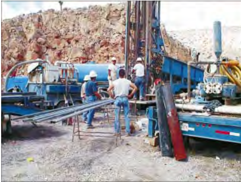
Drilling of well ER-OV-03c near Beatty Wash on the eastern side of Oasis Valley study area (Photograph by Douglas Trudeau, U.S. Geological Survey)
