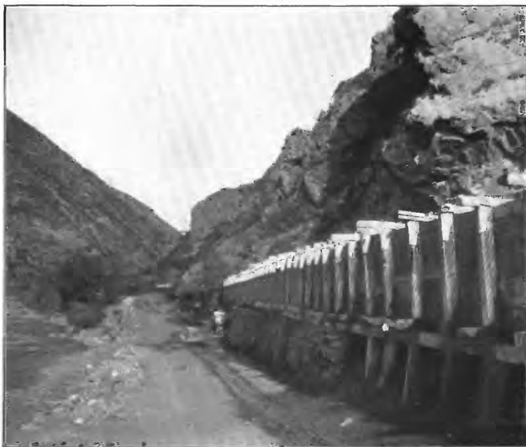
A. LOWER END OF FLUME IN WEST CANAL BRANCH OF BEAR RIVER CANAL, UTAH.
