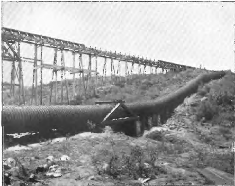
A. OLD FLUME AND NEW REDWOOD STAVE PIPE REPLACING IT, REDLANDS CANAL, CALIFORNIA.
