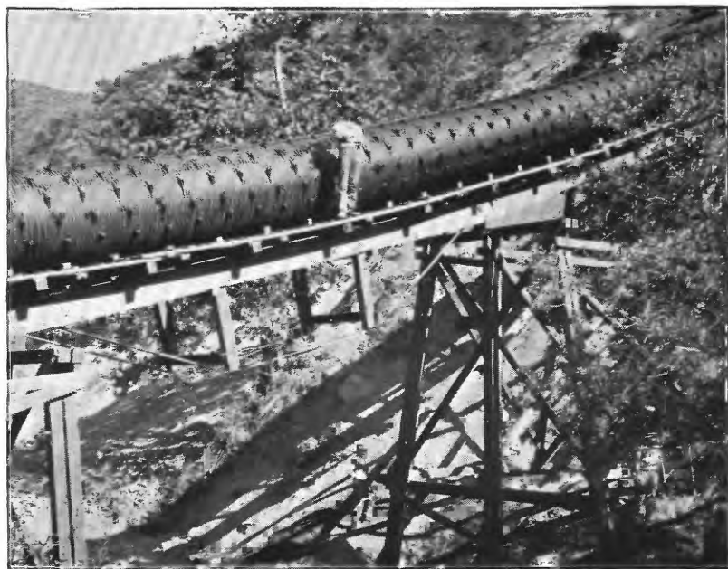
B. REDWOOD STAVE PIPE UNDER 160 FEET HEAD, SANTA ANA CANAL, CALIFORNIA.
