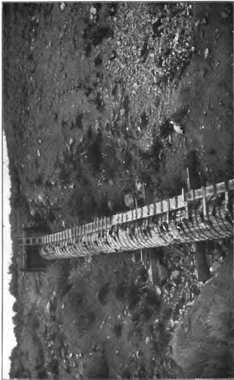
STAVE PIPE OF ELECTRIC-LIGHT WORKS AT BRIGHAM, UTAH.
