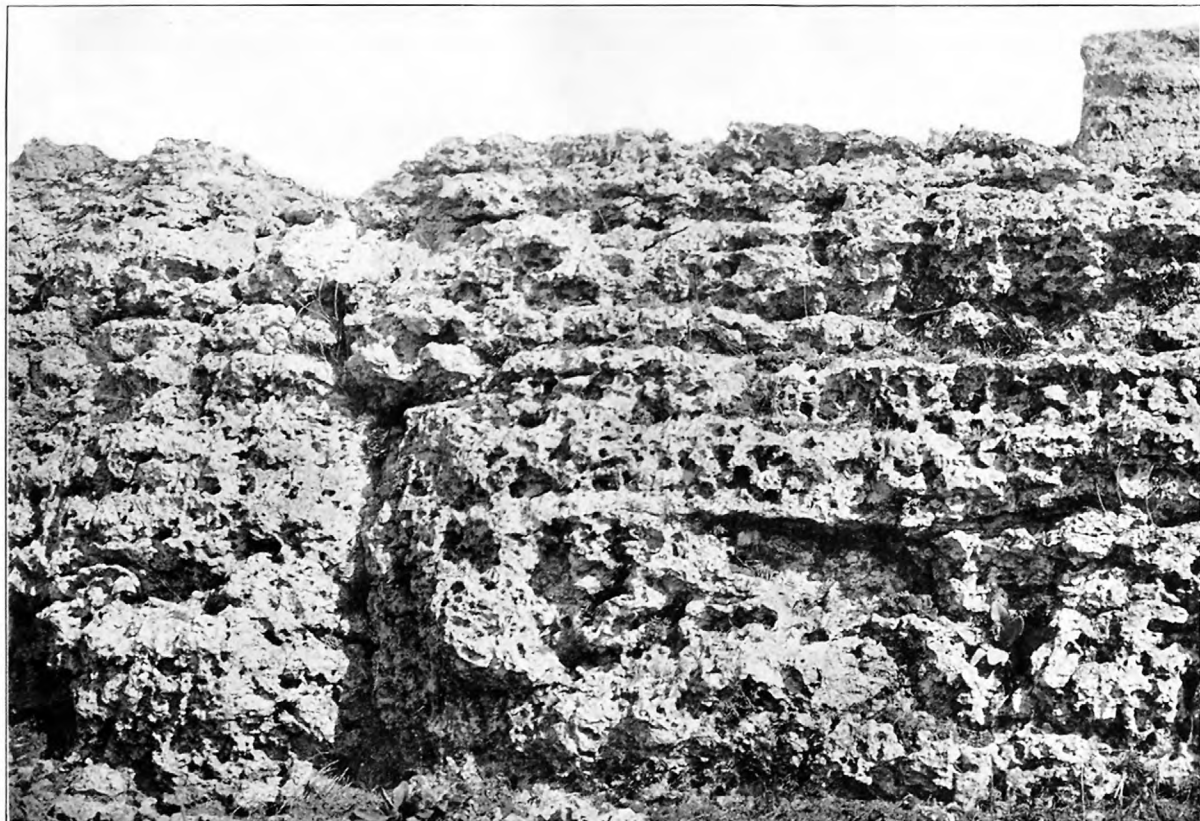
WEATHERED SURFACE OF GALENA DOLOMITE NEAR ROCKDALE, IOWA.
