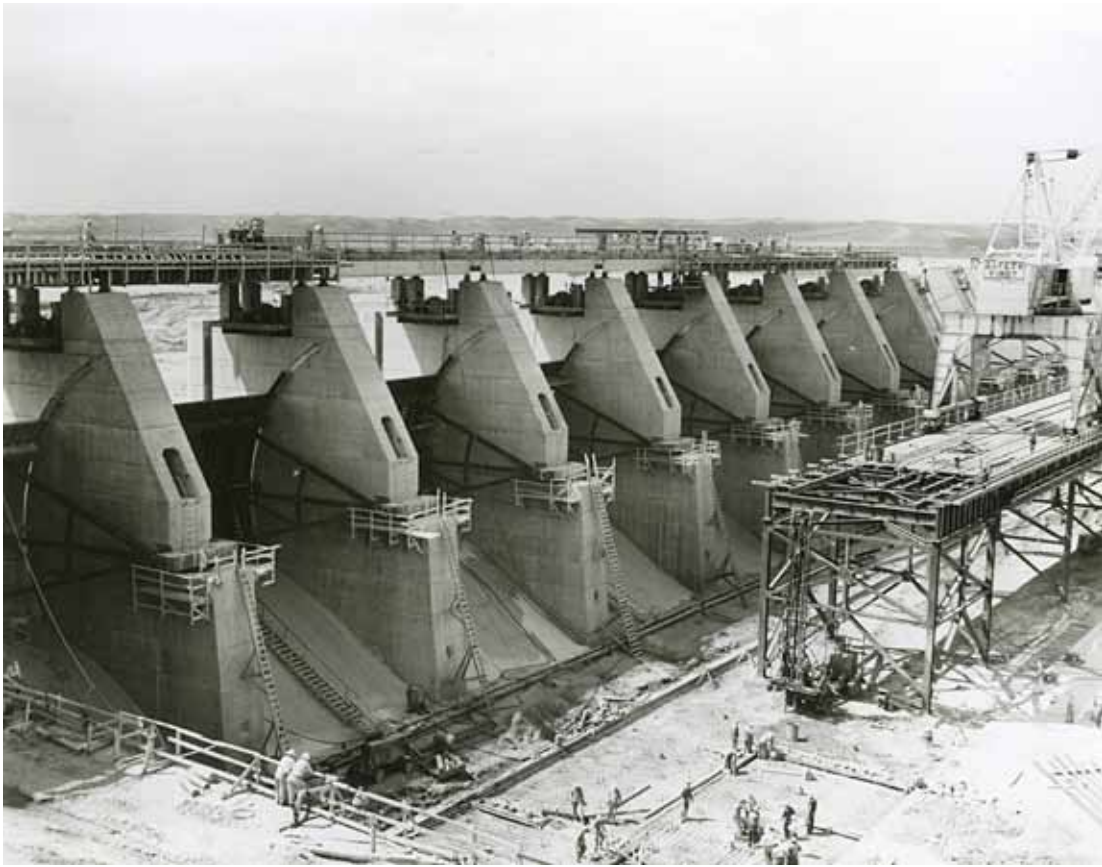
Figure 10. Construction of Gavins Point Dam, circa 1961 (source: U.S. Army Corps of Engineers).
