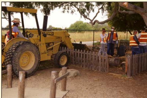
D. Substrate removal during remediation of daycare facility in southern California following infection of children with B. procyonis from rooftop latrine. (Photo by William J. Murray)
