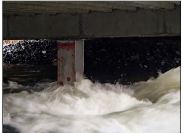
Pier hydraulics at Red Cloud River near Kodiak, Alaska, November 2018. Photograph by Paul Schauer, U.S. Geological Survey.
