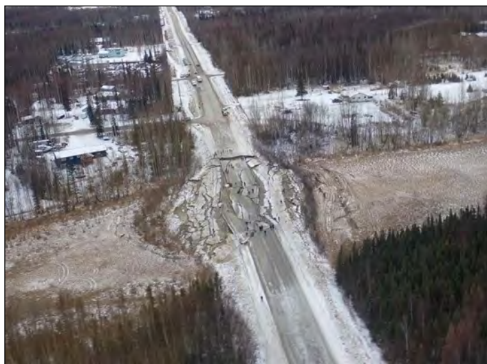
Lateral spreading triggered by the 2018 Anchorage earthquake damaged Vine Road near Wasilla in south-central Alaska. Many failures of engineered materials happened on or adjacent to saturated lowlands filled with organic sediment, silt, or sand. Photograph by Rob Witter, U.S. Geological Survey.
