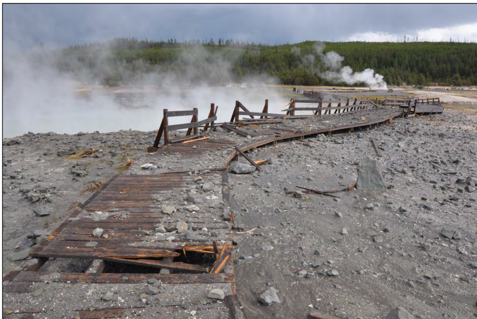
Figure 24. View looking east, toward the Firehole River and Biscuit Basin parking lot, of boardwalk that was damaged during the July 23, 2024, explosion from Black Diamond Pool, which is the steaming area located to the immediate left of the boardwalk. Photograph by Mike Poland, U.S. Geological Survey, September 3, 2024.
