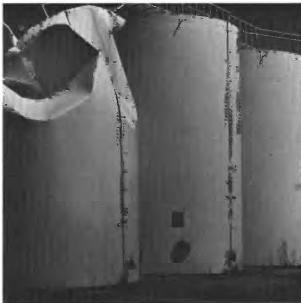
Figure 15.- Damaged cylindrical metal wine-storage tanks at Los Nogales Winery in Cauçete, 80 km southwest of epicenter. Tank at left apparently imploded; vertical steel anchor ties at base were severed, and tank wall at the base buckled. Third tank from the left was similarly damaged at its base; other tanks sustained little or no damage.
