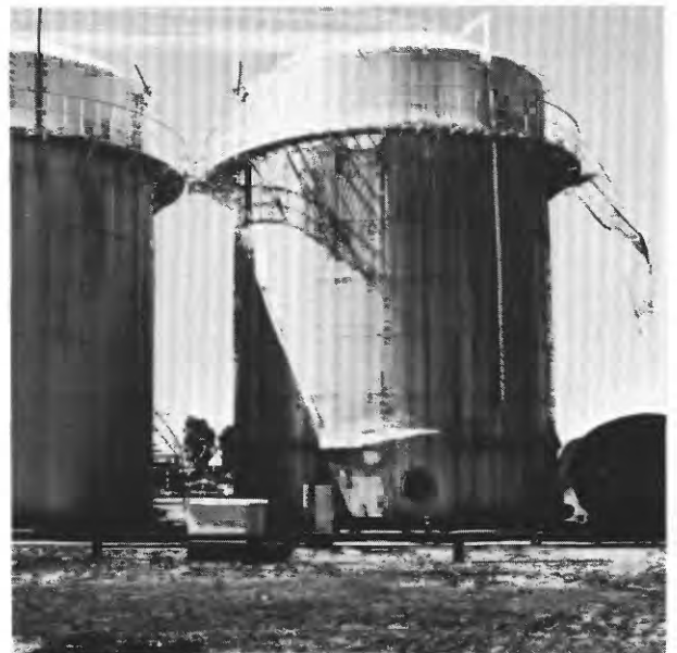
Figure 11.- Damaged metal wine storage tanks at Covic Winery in Media Agua, 117 km southwest of epicenter. Many steel anchor ties at base of both tanks failed in tension or shear.
