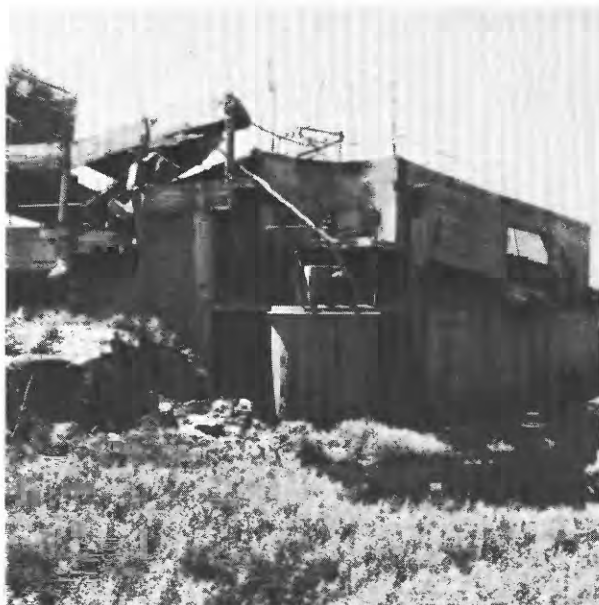
Figure 14.- Collapsed reinforced concrete wine-storage facility at Segura Winery in Cauçete, 80 km southwest of epicenter.
