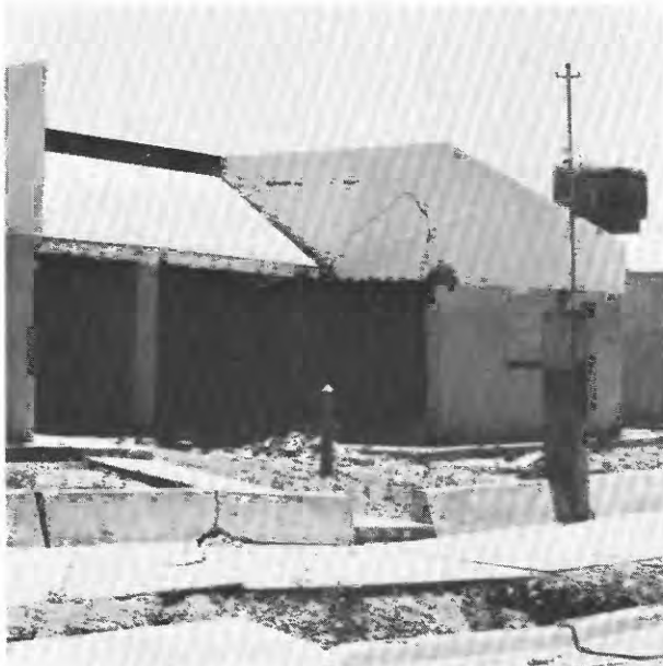
Figure 17.- Damaged one-story masonry-wall house in new development in Cauceca caused by liquefaction. House is located near vertical offset in road pavement shown in figure 16.
