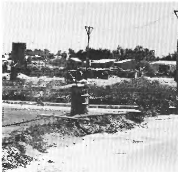
Figure 16.- Subsidence due to liquefaction at a new housing development in Caucete, 80 km southwest of epicenter. Road surface to right of vertical offset subsided 35 cm.
