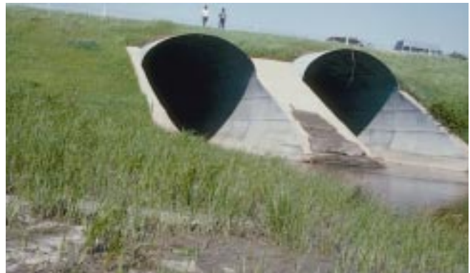
A high-flow event has deposited sediment on the flood plain (foreground) and on the lower part of the concrete structure separating these two culverts on Two Rivers near Northcote, Minnesota.
