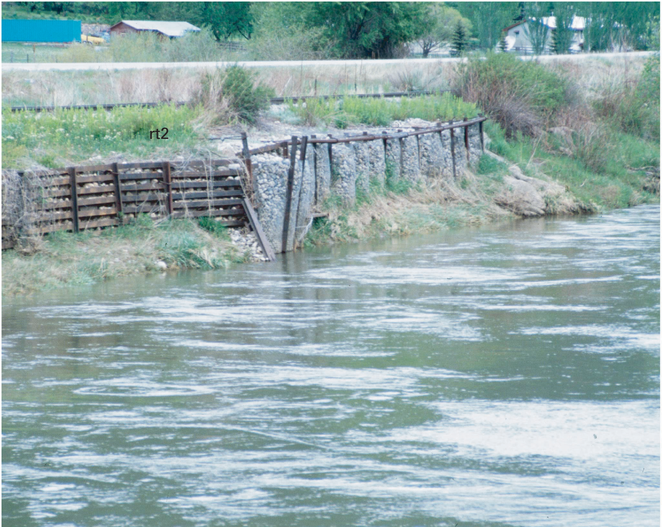
17. Terrace deposits (t). View looking northwest at stabilization works on a rt2 terrace cut bank in the lower Animas River valley.
