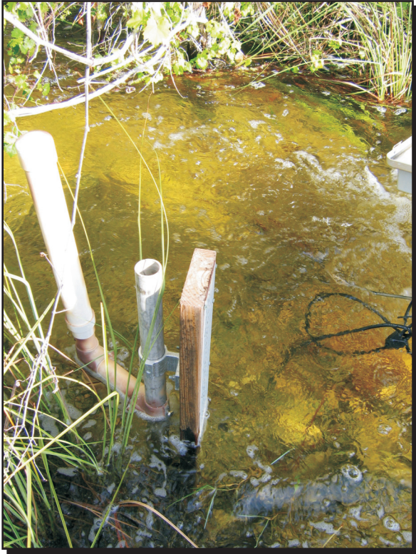
Figure 5. Installed Global Water Instrumentation pressure sensor. The polyvinyl chloride (PVC) pipe behind the staff plate housed the pressure sensor.
