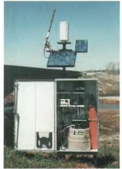
Streamflow-gaging/water-quality sampling equipment typical of Phase II sampling sites.
