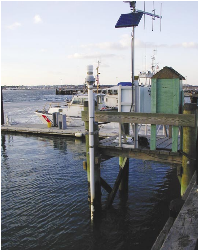
Figure 4. U.S. Geological Survey tide gage at Cape May Harbor in Cape May, N.J., which transmits tide elevation and meteorologic data via satellite and VHF radio for emergency management and other purposes. (Photograph by Peter B. Reilly, U.S. Geological Survey)
