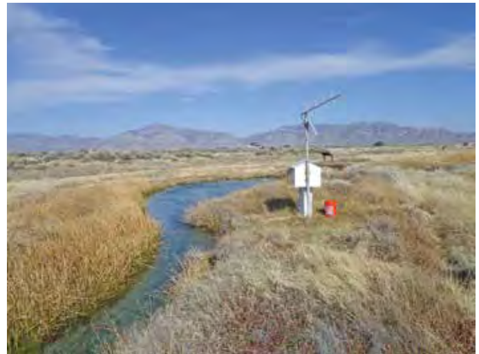
Figure 2. Streamflow station at Hot Creek near Sunnyside, Nevada.
