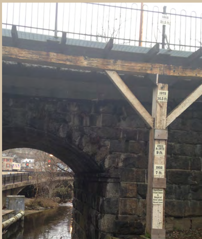
Figure 3. Flood markers at bottom of Main Street at railroad trestle, Ellicott City, Maryland. Photograph by John C. Hammond, U.S. Geological Survey, December 5, 2014.
