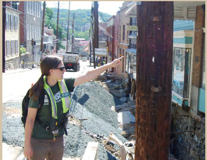
Figure 4. The approximate high-water elevation and damage to sidewalks along Main Street in Ellicott City, Maryland, in the aftermath of the July 30, 2016, storm and flood. Photograph by Eric L. Boyd, U.S. Geological Survey, August 5, 2016.
