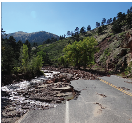
Flood damage on Left Hand Canyon highway. Photograph by Geoffrey Plumlee.
