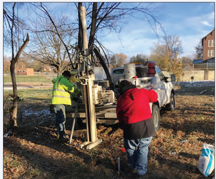
Figure 9. U.S. Geological Survey personnel installing a piezometer at a St. Louis, Missouri, demolition site. Photograph by David Heimann, U.S. Geological Survey.
