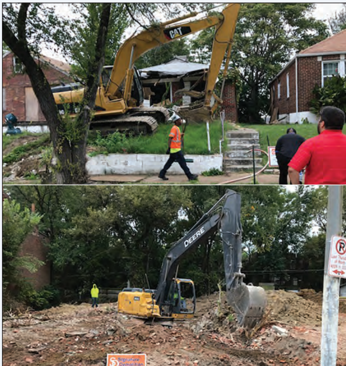
Figure 7. Vacant building deconstruction in St. Louis, Missouri, removes, A , impervious surfaces and, B , replaces them with pervious soil that can retain stormwater and reduce runoff. Photographs by David Heimann, U.S. Geological Survey.
