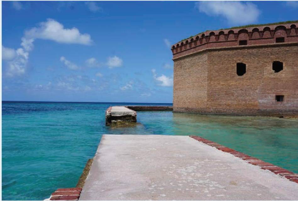
Figure 3. View of collapsed moat wall at Dry Tortugas National Park (DRTO), Florida, after Hurricane Irma, which made landfall in southern Florida in 2017. Photograph by D. Diaz, National Park Service, October 2020.
