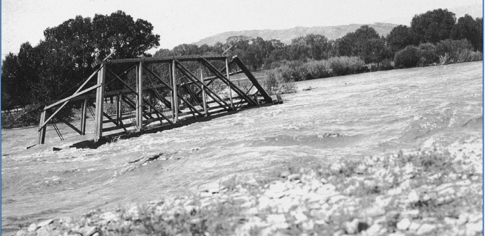
The 1918 Yellowstone River flood caused the Harvat Bridge washout in Livingston, Montana (image number 2011.010.0395 provided by the Yellowstone Gateway Museum, used with permission).
