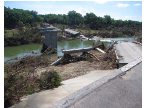
Figure 2. Bridge destroyed by flooding of the Blanco River at Fischer Store Road near Wimberley, Texas, in May 2015. Photograph taken June 1, 2015. Courtesy of U.S. Geological Survey Oklahoma-Texas Water Science Center.
