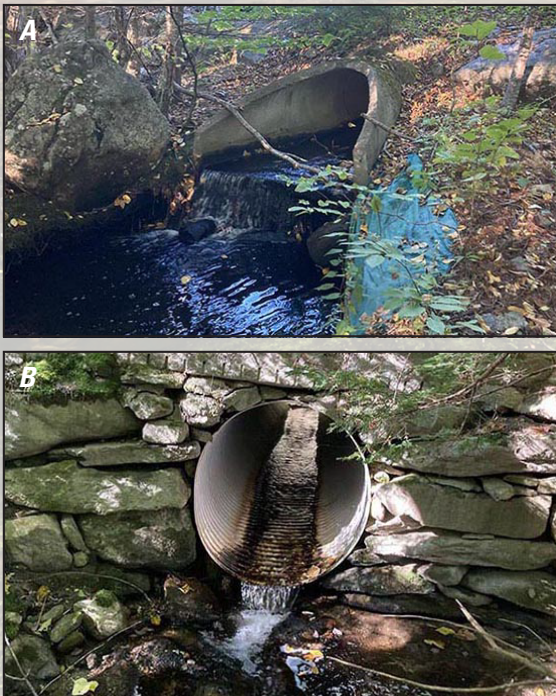
Figure 1. Photographs showing A , Pearl Hill Brook at Mill Creek Drive in Ashby, Massachusetts, on October 1, 2021, where the drop at the outflow of the culvert may impede aquatic organism passage, and B , an unnamed tributary to Trapfall Brook at Harris Road in Ashby, Massachusetts, on October 1, 2021, where the shallow water in the culvert (and the drop at the outflow) may impede aquatic organism passage. Photographs by Brian Nelson, U.S. Geological Survey.
