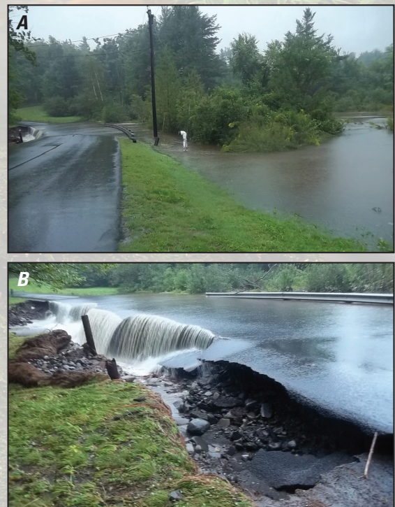
Figure 2. Photographs showing Clesson Brook flooding the culvert and road on Pond Road in Hawley, Massachusetts, on August 28, 2011. A , The flooded culvert and road about 200 feet away. B , The undersized culvert did not allow this flood flow to pass through the structure. Photographs by the University of Massachusetts Amherst, River Smart Communities, used with permission.
