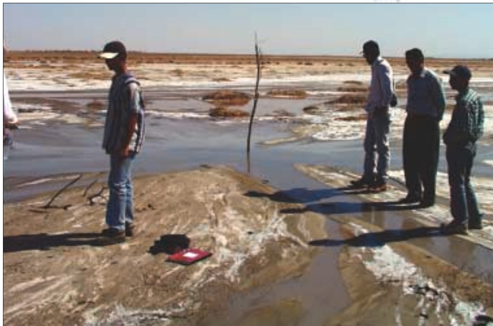
Figure 1. Close-up view of liquefaction taken several weeks after the Bhuj earthquake near the village of Umedpar. Shaking caused the saturated soils and sands to lose their strength and compact, raising the water pressure until water and sediment erupted on the surface as sandblows. As the salty water dries, a white salty crust is left behind. This part of the epicentral area, known as the Banni Plain, is adjacent to an inlet to the sea (the Great Rann of Kutch) that floods annually. The extremely flat topography suggests that the rates of geologic activity must be very low because high rates build mountains and other topographic relief. (Photo courtesy of Gary Patterson, Center for Earthquake Research and Information, Memphis, Tenn.)
