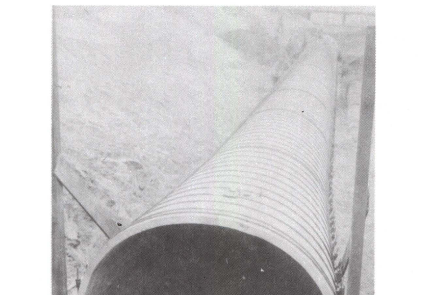
Wooden inverted pipe construction of a canal siphon under Power Creek, Kern County, in the late 1800's. (City of Bakersfield, Department of Water.)
