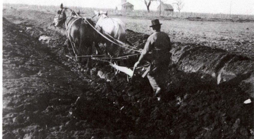
Ditching with a plow in the early 1900's. A canal bottom is scarified to prepare for excavation. (Woodbridge Irrigation District.)
