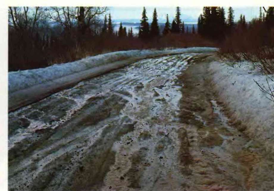
Figure 3c. -- Erosion of road by melt water during the spring (Spain Drive near Potter Creek, April 1980).
