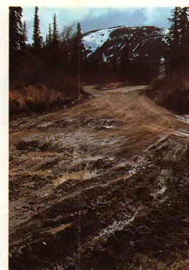
Figure 3d. -- Road damaged by poor drainage and high water table during the spring (Carl Street near upper Little Rabbit Creek, May 1980).
