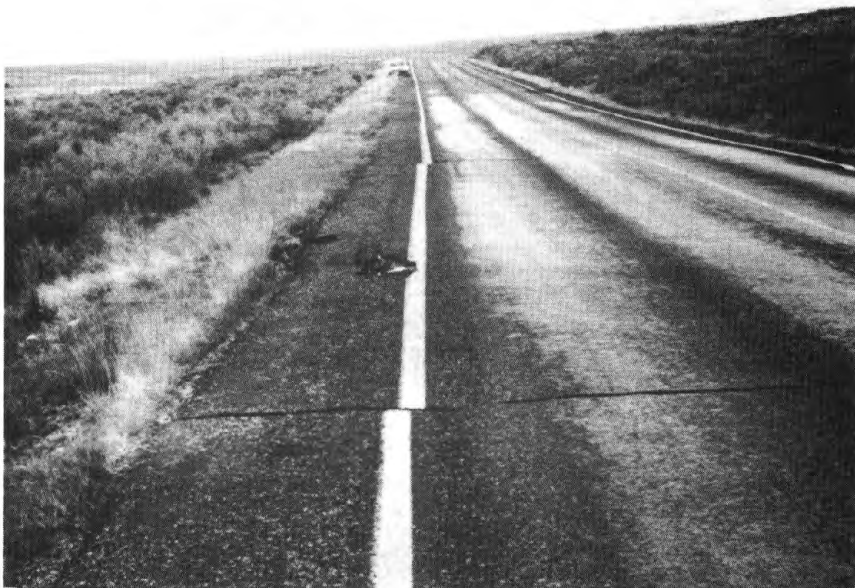
Figure 9. Displacement of Highway 93 south of Whiskey Springs due to lateral spreading (site 2). Highway slabs nearest the camera moved downslope to the left. View looking north.
