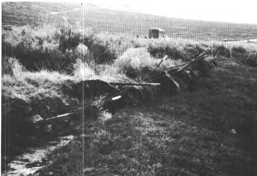
Figure 7. Buckled and overturned sod at the toe of lateral spread mapped on Fig. 5. This disruption occurred below damaged section of Highway 93 where fissures above highway and lateral displacement of highway was greatest (site 2).
