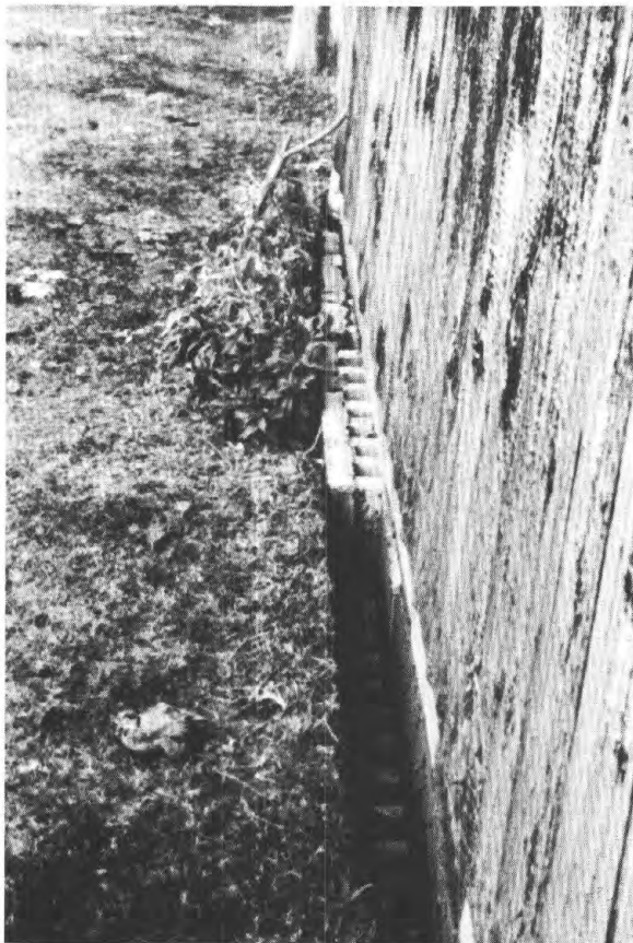
Figure 2B. Damaged perimeter foundation at back of house.
