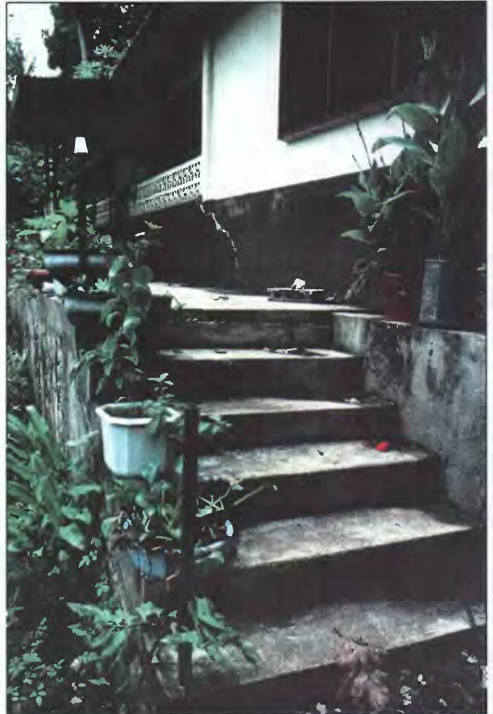
Figure 8. Fractures in foundation of house and steps resulting from movement on incipient rotational slump near Tamwarohi.
