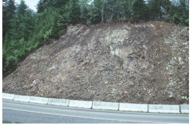
B) Landslide in slate of the Anakeesta Formation on Rt. 441, west of Newfound Gap.
