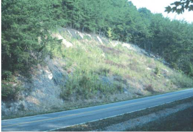
A) Landslide in quartzite regolith along the Foothills Parkway, east of Cosby.
