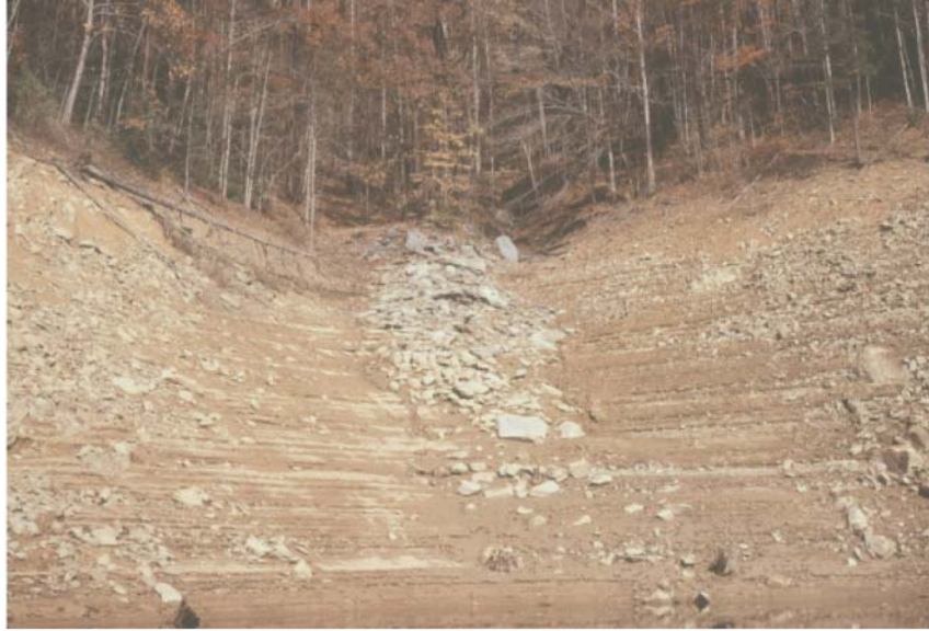
Fig. 52- A) Draw-down of Fontana Lake (horizontal water lines), reveals boulder debris concentrated in hillslope depressions
