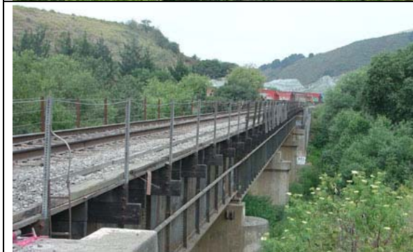
Figure 2-20. The original railroad bridge over the Pajaro River was heavily damaged by the 1906 earthquake. The bridge straddles a strand of the San Andreas Fault, which caused minor rotational offset of the bridge during the 1906 earthquake. The area also experienced heavy shaking during the 1989 earthquake. Piles of gravel from the Logan Quarry are in the distance.
