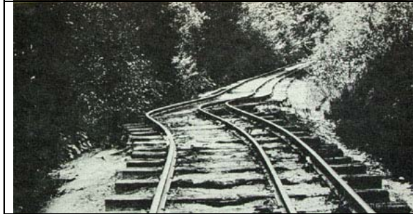
Figure 3-7. Damage to the railroad track between Wrights Station (near the tunnel) and Alma caused by the 1906 earthquake. Both historic settlements and the rail line no longer exist. The gravel road now follows the rail path. The photograph is from the Lawson Report.
