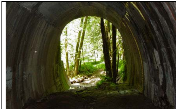
Figure 3-6. View looking out of the west end of Wrights Tunnel toward Los Gatos Creek. The tunnel is now full of leaking cracks that are feeding a small stream flowing from the mouth of the passage.
