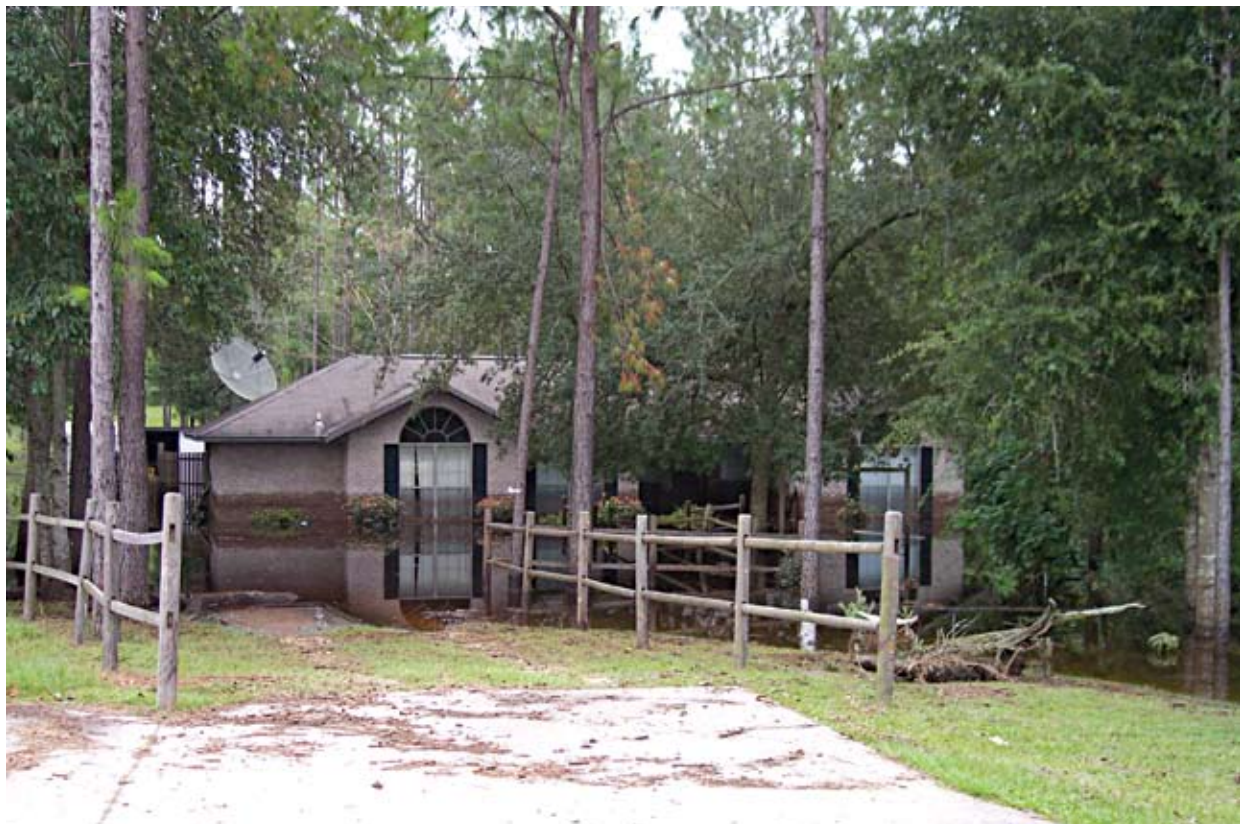
Figure 5. House on State Road 47 near Rose Sink (Columbia County), September 11, 2004. Note the high water mark on the house. Image courtesy of Al Sandrik of the National Weather Service.
