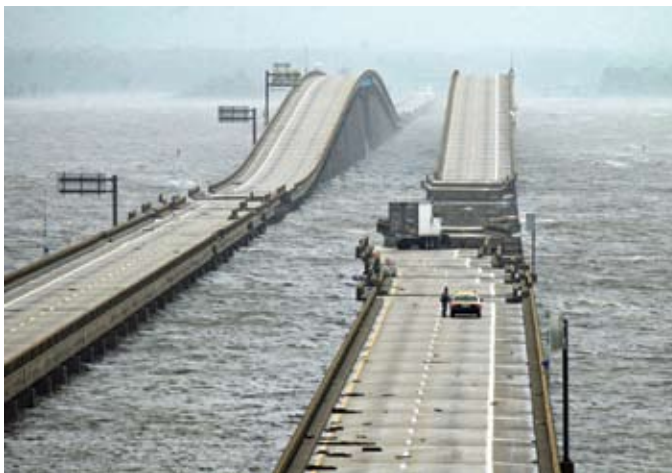
Figure 7. Interstate 10 (I-10) bridge over Escambia Bay; bridge sections displaced laterally and vertically. Photo courtesy Pensacola News Journal, Copyright 2004.
