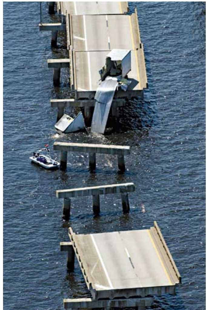
Figure 8. Semi truck hanging off a broken section of the I-10 bridge, Escambia Bay. Photo courtesy Pensacola News Journal, Copyright 2004.
