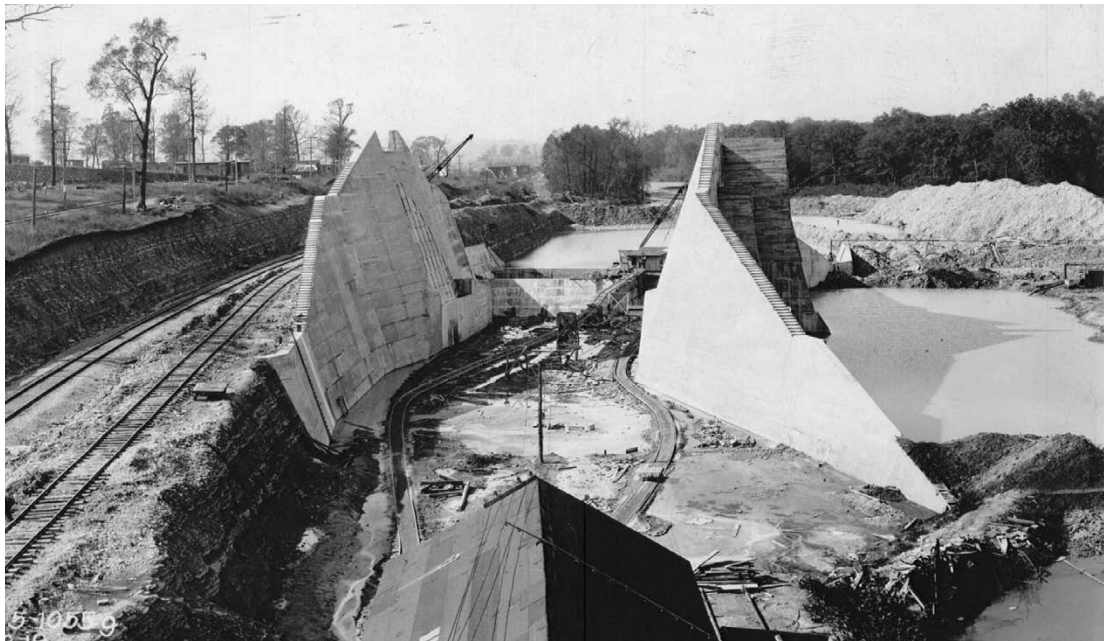
Construction of the outlet at Huffman Dam spillway. (Photo furnished by the Miami Conservancy District, copyright 1913–2009, all rights reserved; reproduced with permission.)
