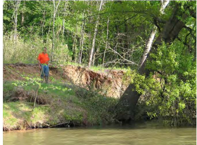
Figure 7. A recent (summer 2005) bank failure near Hamilton, N.C.
