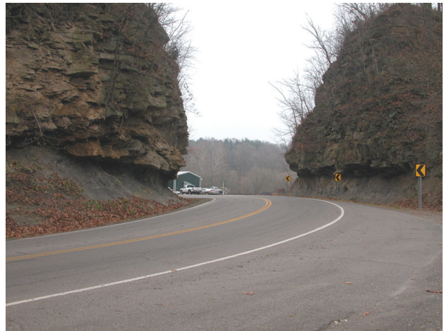
Figure 4. Outcrop of the Grafton sandstone of Hennen and Reger (1913) in Brooke County in West Virginia's northern panhandle. The gap in this narrow ridge was created when one of two of the oldest tunnels on the western slope of the Appalachians was daylighted.
