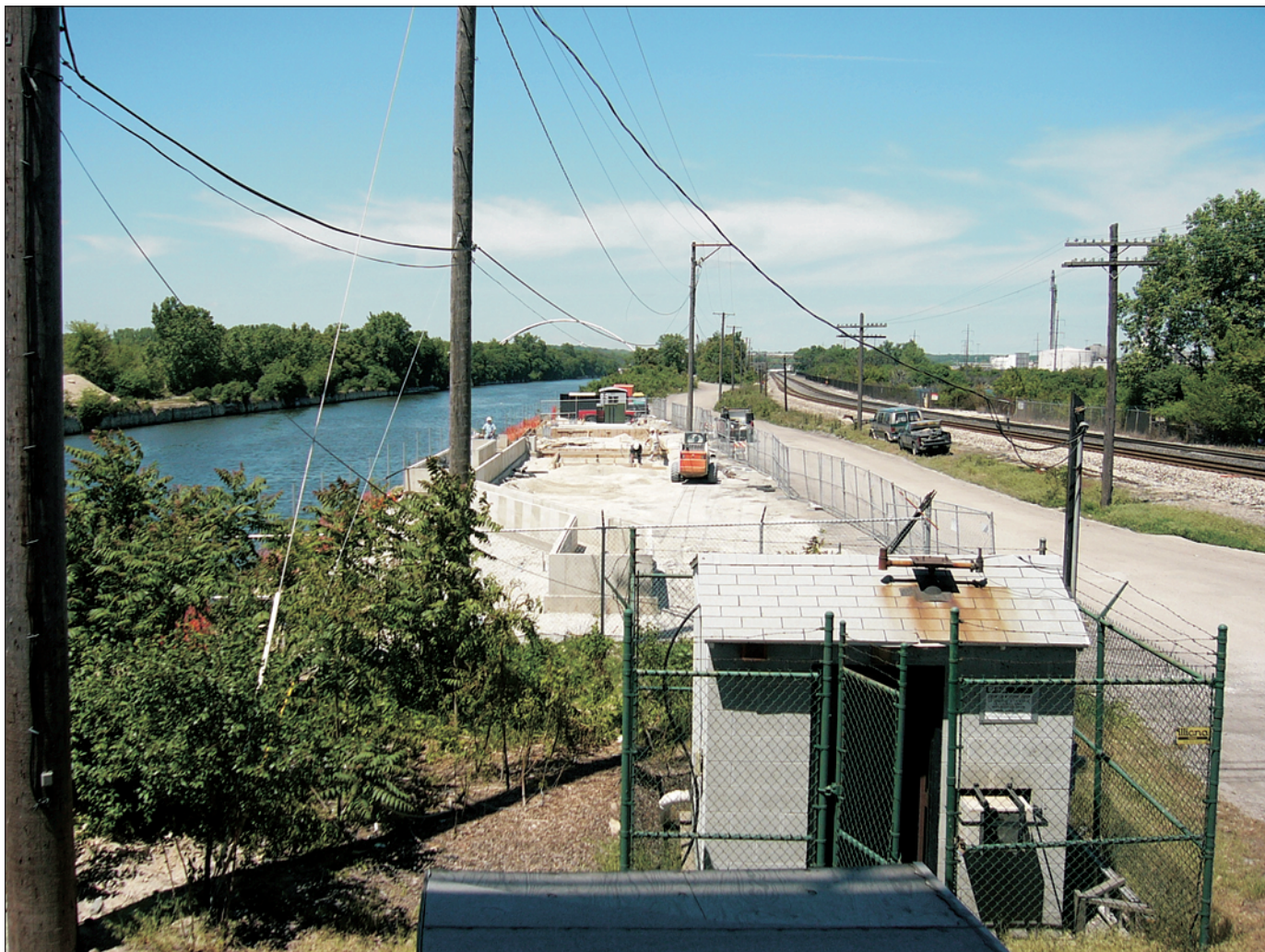
Figure 9. Photograph showing proximity of electric dispersal barrier 2A construction activities to the streamflow-gaging station on the Chicago Sanitary and Ship Canal at Romeoville, Illinois.
