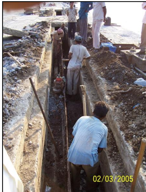
Figure 12. Photograph of utility and crane rail trench filled with debris and utilities damaged by the 2004 Sumatra Tsunami in Port Blair, India (photograph by Martin Eskijian).
