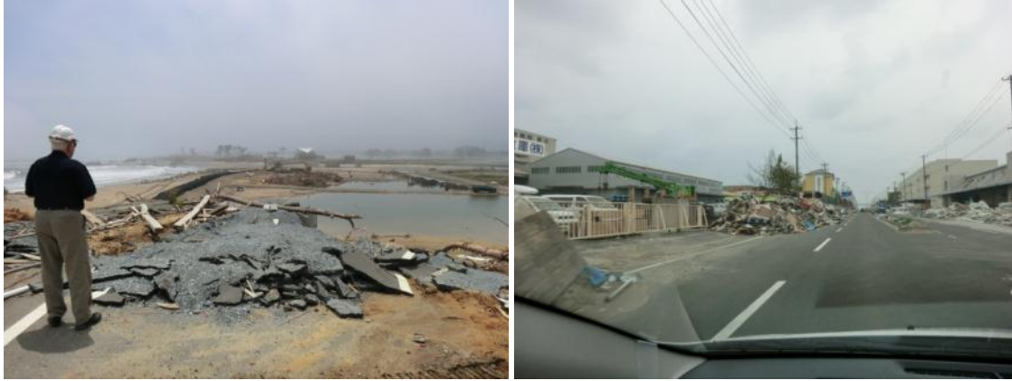
Figure 61. Photographs of tsunami damage from the 2011 Tohoku, Japan, tsunami: Left, About 1 mile of Route 38 north of Shinchi was washed away by the 2011 Tohoku tsunami. Right, Roads throughout the Port of Sendai were largely undamaged despite high currents and depths; they had no embankments that could generate scouring vortices. (Photographs by Keith Porter.)
