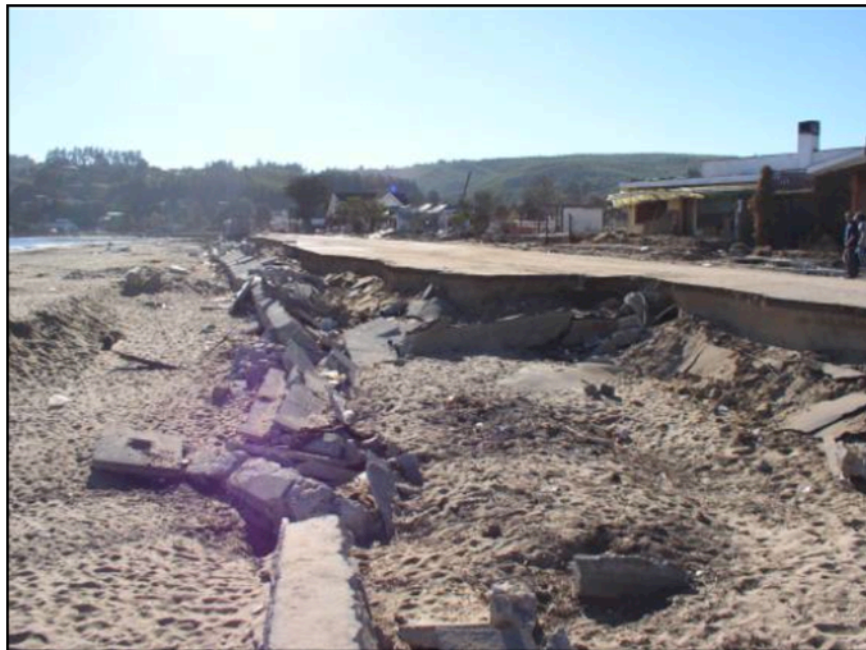
Figure 10. Photograph of seawall and road damaged in Chile Tsunami of 2010 (photograph from American Society of Civil Engineers, Coasts, Oceans, Ports, and Rivers Institute, 2005).
