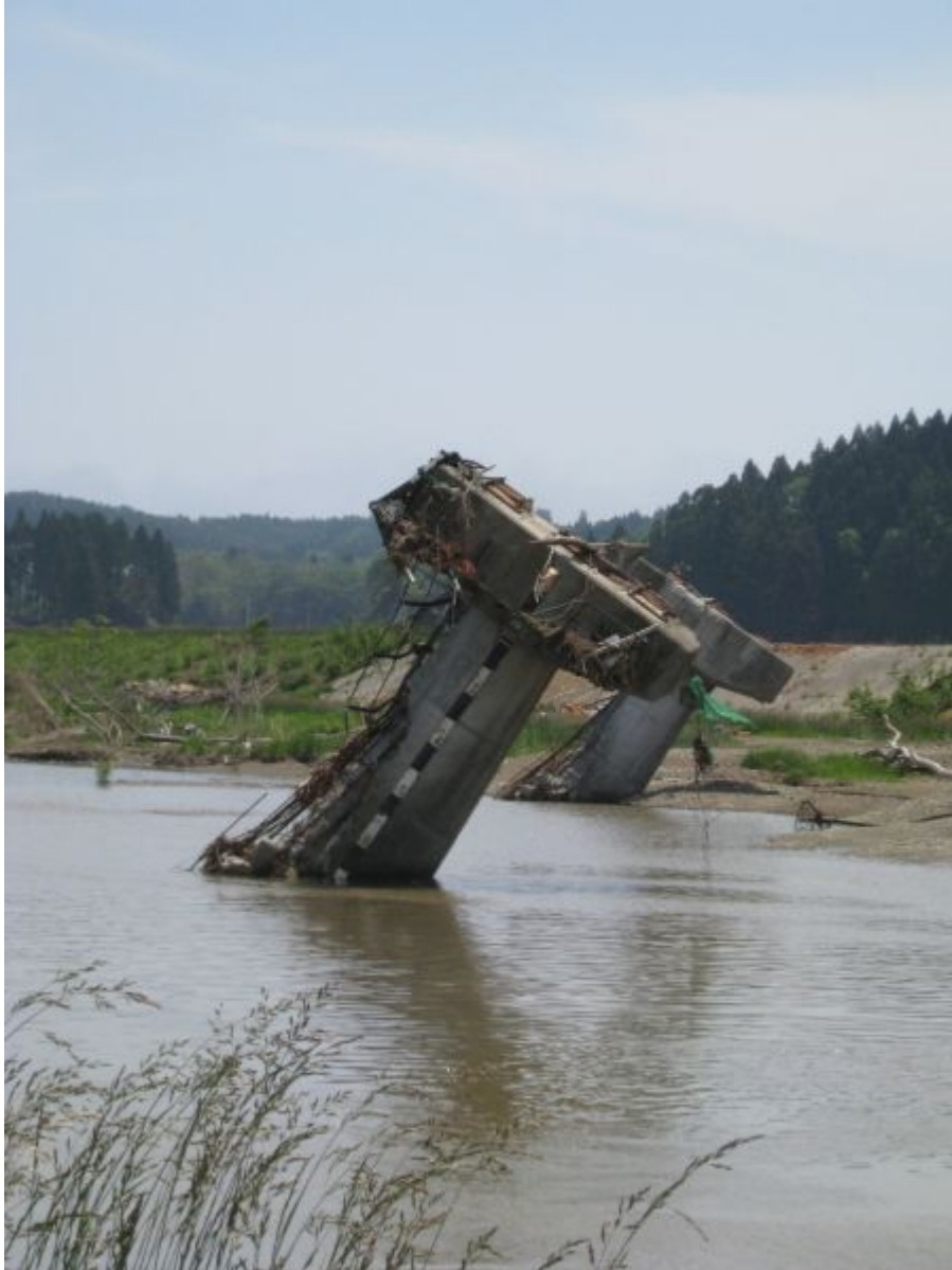
Figure 70. Photograph of damaged piers of the JR Rail Viaduct crossing the Tsuya River, Japan, after the 2011 Tohoku tsunami (photograph by Shideh Dashti).
