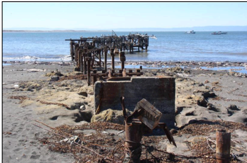
Figure 18. Photograph of pier deck removed in Chile Tsunami of 2010 (photograph from American Society of Civil Engineers, Coasts, Oceans, Ports, and Rivers Institute, 2010).
