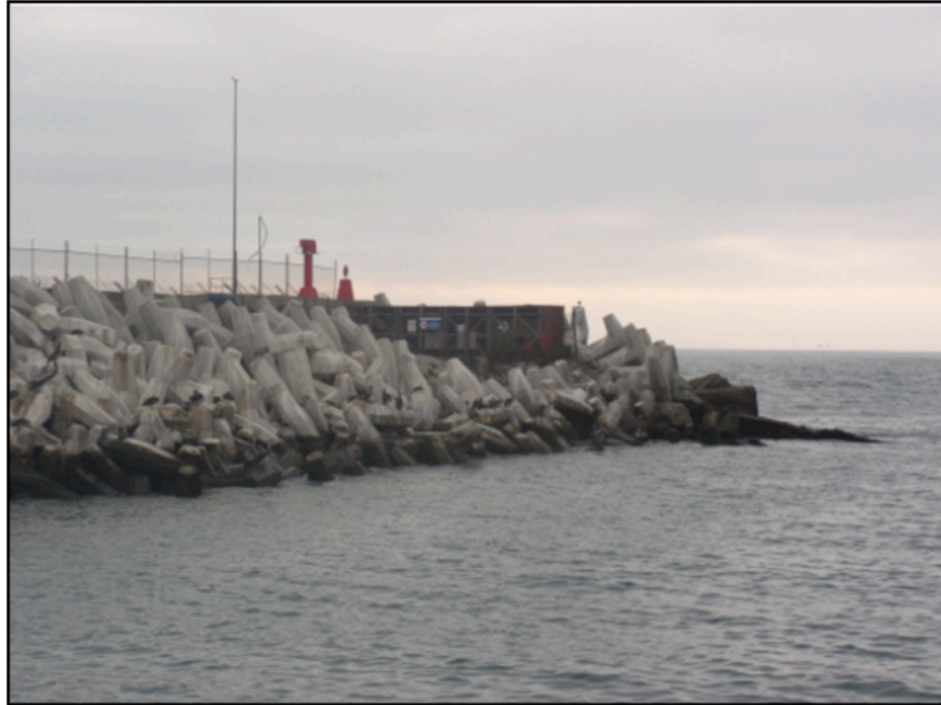
Figure 9. Photograph of breakwater damaged in Chile 2010 Tsunami (photograph from American Society of Civil Engineers, Coasts, Oceans, Ports, and Rivers Institute, 2005).
