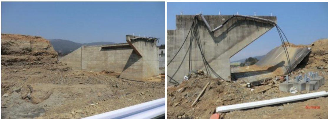
Figure 60. Photographs of embankment scour at Route 45 bridge (Takada Bypass) over Route 141 (Hamaiso Highway) due to the 2011 Tohoku tsunami (photographs by Charles Scawthorn).
