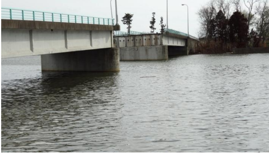
Figure 65. Photograph of damage from a barge impact on the Jokawa Bridge over the Higashimatsushima River in the 2011 Tohoku, Japan, tsunami that destroyed the middle span and damaged the other spans (photograph by Junichi Hoshikuma).
