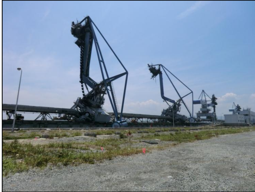
Figure 15. Photograph of container cranes collapsed due to tsunami current forces at Port of Shinchi, Japan, following the 2011 Tohoku tsunami (photograph by Keith Porter).
