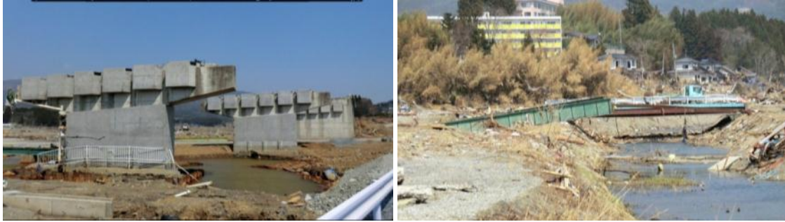
Figure 63. Photographs of bridges whose superstructures were pushed or floated off their piers in the 2011 Tohoku, Japan, tsunami (photographs by Charles Scawthorn).
