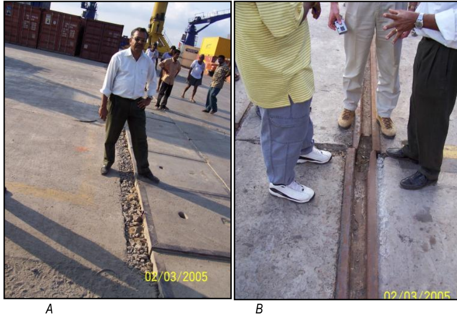
Figure 11. Photographs of damage from 2004 Sumatra Tsunami in Port Blair, India. A , Differential settlement between pile supported wharf and backfill area in Port Blair, India. B , Container crane rail misalignment. (Photographs by Martin Eskijian).
