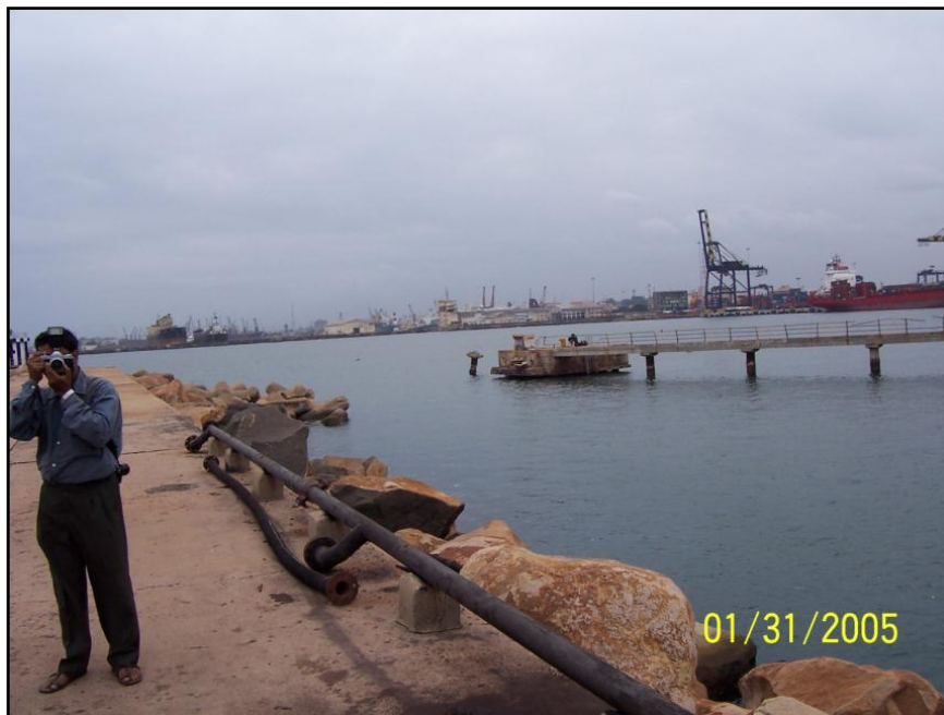
Figure 7. Photograph of Port of Chennai, India—two mooring dolphins missing after the 2004 Sumatra Tsunami (photograph by Martin Eskijian).
