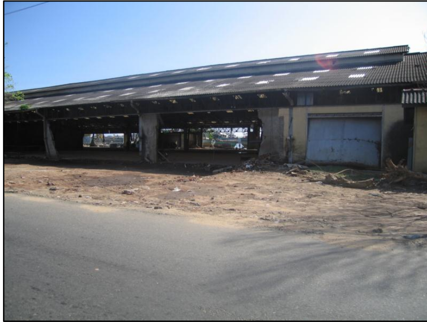
Figure 17. Photograph of Sri Lankan Port of Galle warehouse damage during 2004 Sumatra Tsunami (photograph from American Society of Civil Engineers, Coasts, Oceans, Ports, and Rivers Institute, 2005).
