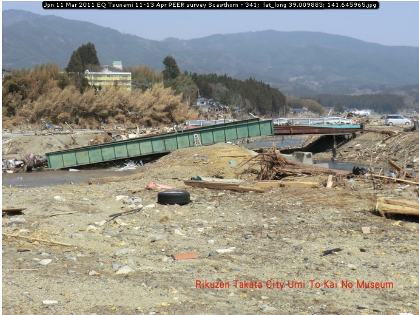
Figure 69. Photograph of displaced steel girder span near Rikuzen Takata after 2011 Tohoku, Japan, tsunami (photograph by Charles Scawthorn).
