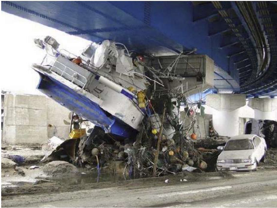
Figure 64. Photograph of example from the 2011 Tohoku, Japan, tsunami of how small craft represent a debris hazard for bridges; the Miyako Bridge across the Hei River in the City of Miyako (photograph by Junichi Hoshikuma).
