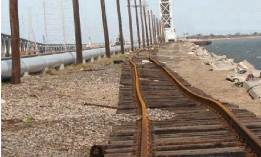
Figure 75. Photograph of track damage from 2008 Hurricane Ike in the United States. Surge depth was about 3 feet above track (photograph by Ross Ruckel).
