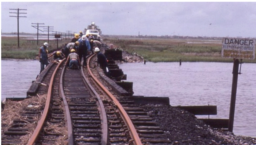
Figure 74. Photograph of open deck trestle damage from 1983 Hurricane Alicia in the United States. Deck shifted by return flow. Surge depth was about 3 feet above track, about 5 feet above bottom of deck. (Photograph by William Byers.)
