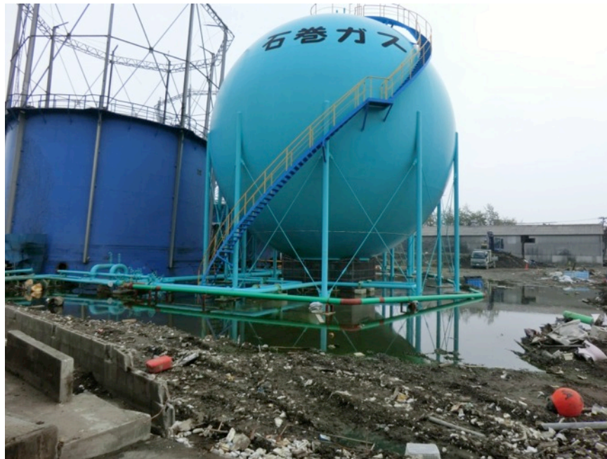
Figure 21. Photograph of pipes whose supports seem to have been undermined by tsunami scour in Ishinomaki, Japan, after the 2011 Tohoku tsunami (photograph by Keith Porter).
