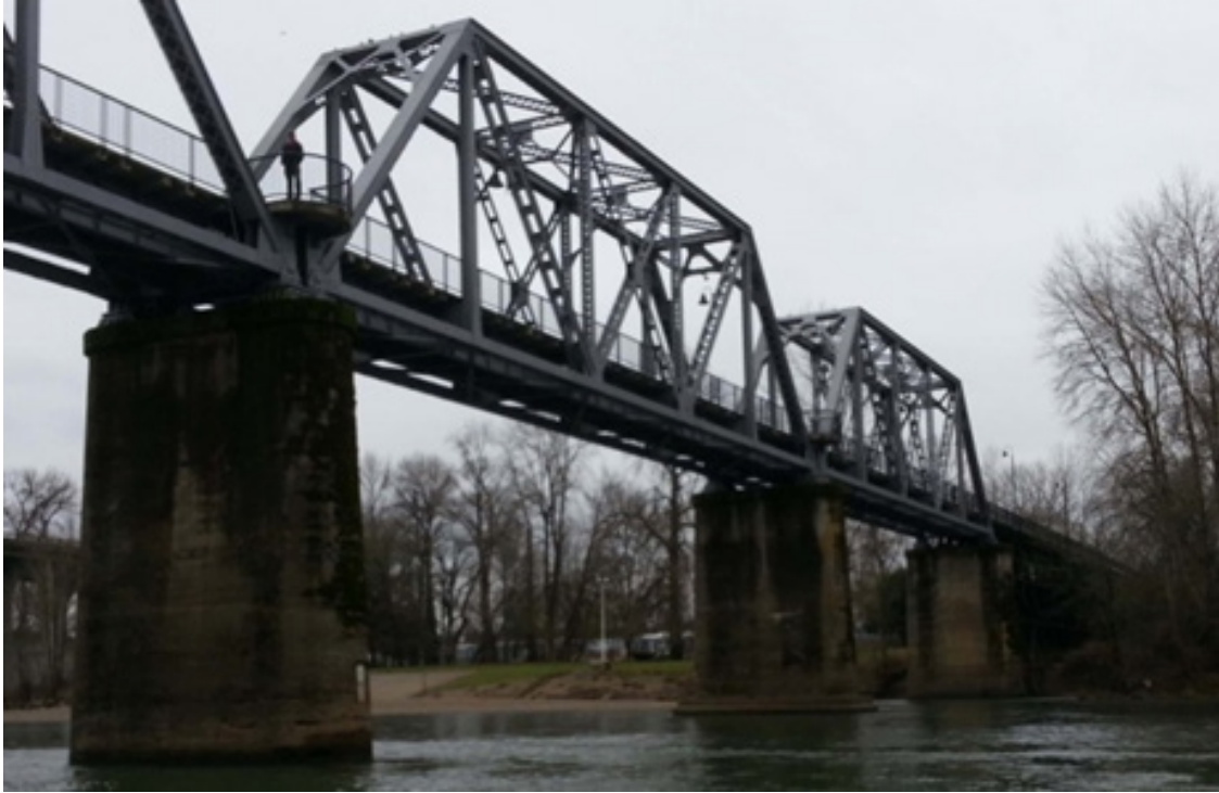
Figure 11. Photograph of Union Street Bridge in Salem, Oregon, 2012. This is an example of the types of bridges crossing the Willamette River that can be used to mount Juvenile Salmon Acoustic Telemetry System (JSATS) monitoring equipment. Photograph taken by Matthew Sholtis, U.S. Geological Survey.
