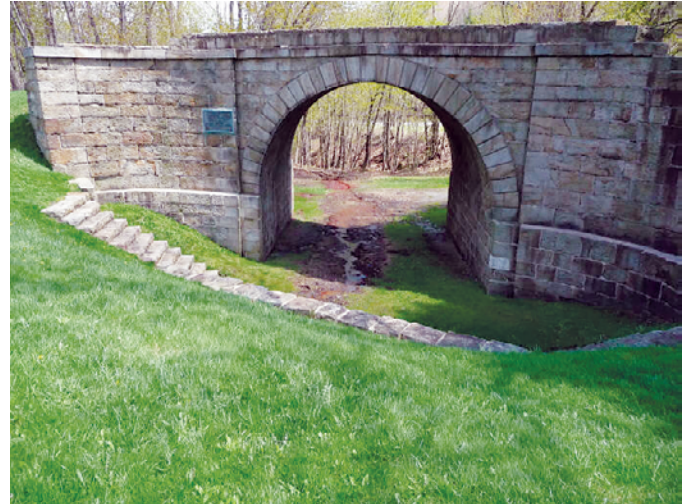
Figure 4. Skew Arch Bridge showing contaminated seepage from the base of the bridge October 10, 2014, at altitude of approximately 2,120 feet NAVD 88. Photograph by Kathy A. Penrod, National Park Service.
